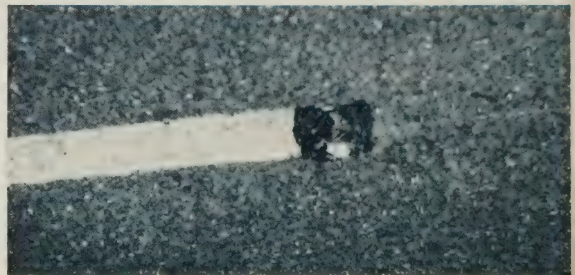
Figure 4.—Pavement damage due to the removal of a raised pavement marker.
