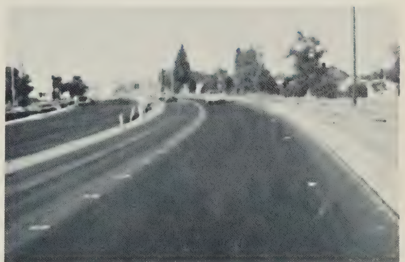
Figure 2.—Raised pavement markers used for centerline and edgeline without paint stripes.
