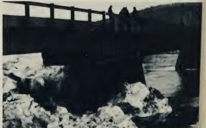
Figure 3.—St. John River Bridge, Allagash, Maine—superstructure has slid 3 ft (1 m) on pier number 4 from its original position. (3)
