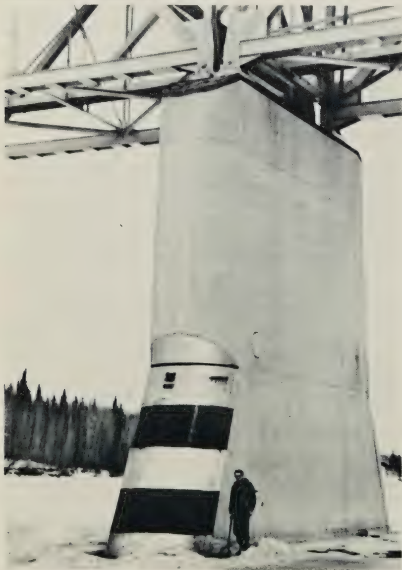
Figure 8.—Load-measuring pier, Hondo Bridge. Painted stripes 3 ft (0.9 m) high enable ice level to be read from photographs. (10) —courtesy, Alberta Department of Highways and Research Council of Alberta
