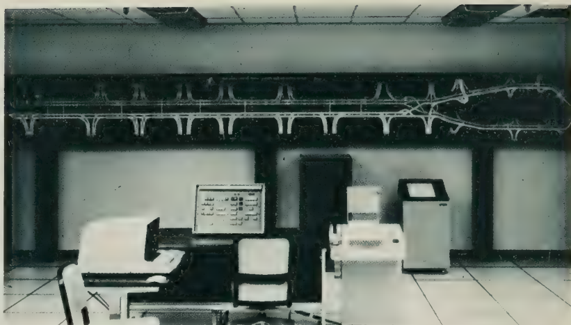
Figure 5.—New Jersey Turnpike System—Traffic Control Center.
