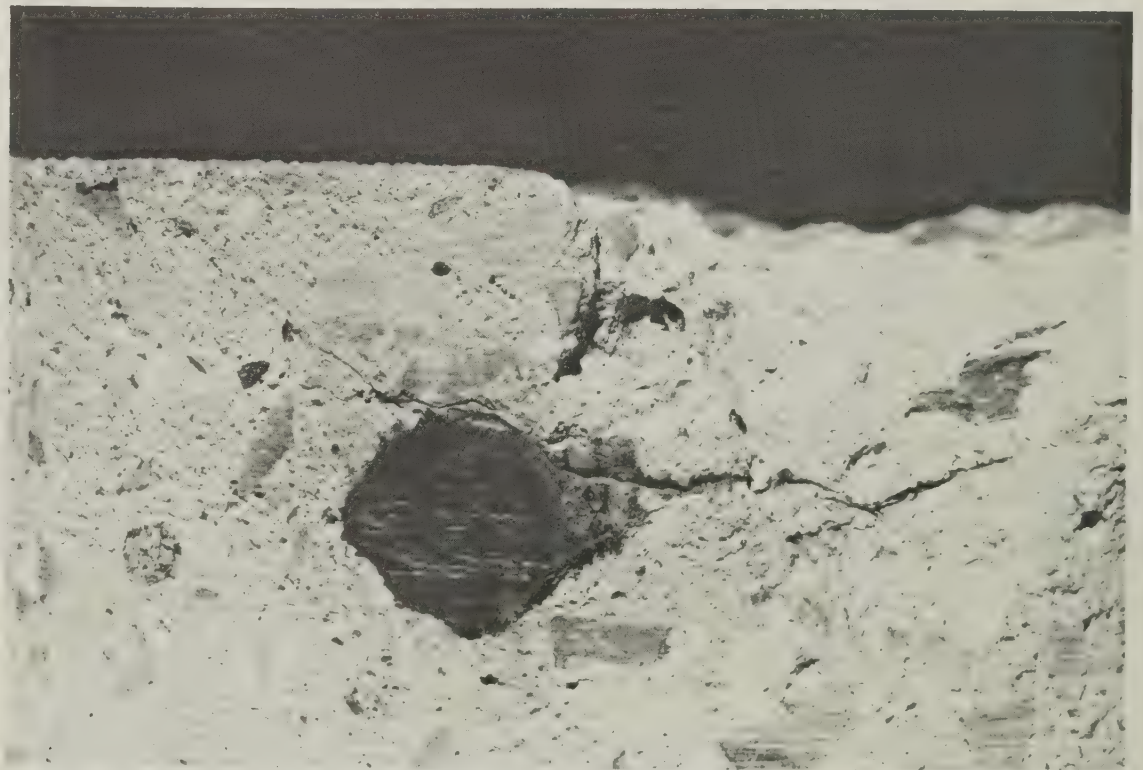
Figure 5.—Corrosion caused concrete cracking.
