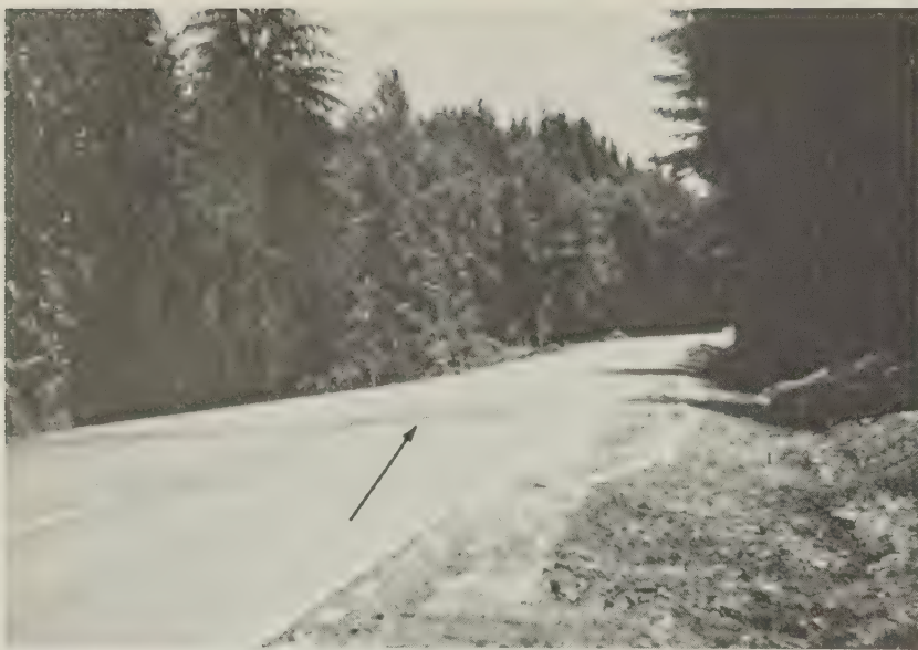
Figure 3.—Preconstruction view of lightweight fill section. Crack line indicates sliding.
