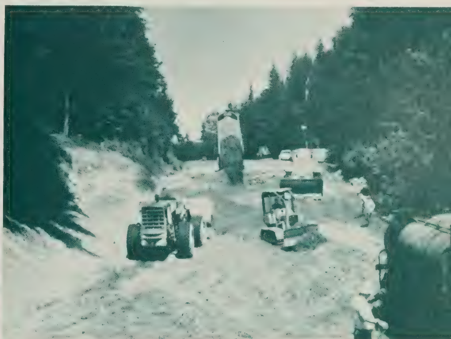
Figure 9.—Sawdust was placed in 1-foot lifts and was compacted with construction equipment in a predetermined pattern.
