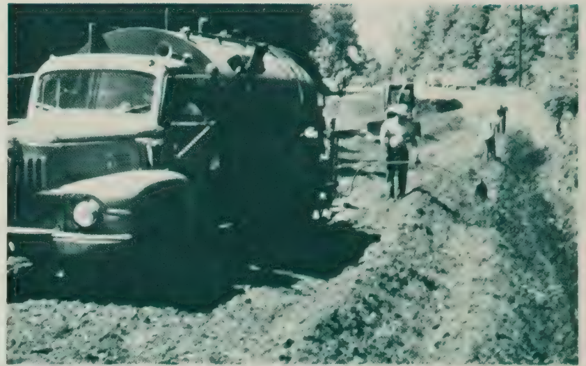
Figure 11.—On the fill slope, an emulsified asphalt sealer was applied with each lift of sawdust while in the background laborers hand mix the wood fibers with the heated asphalt.
