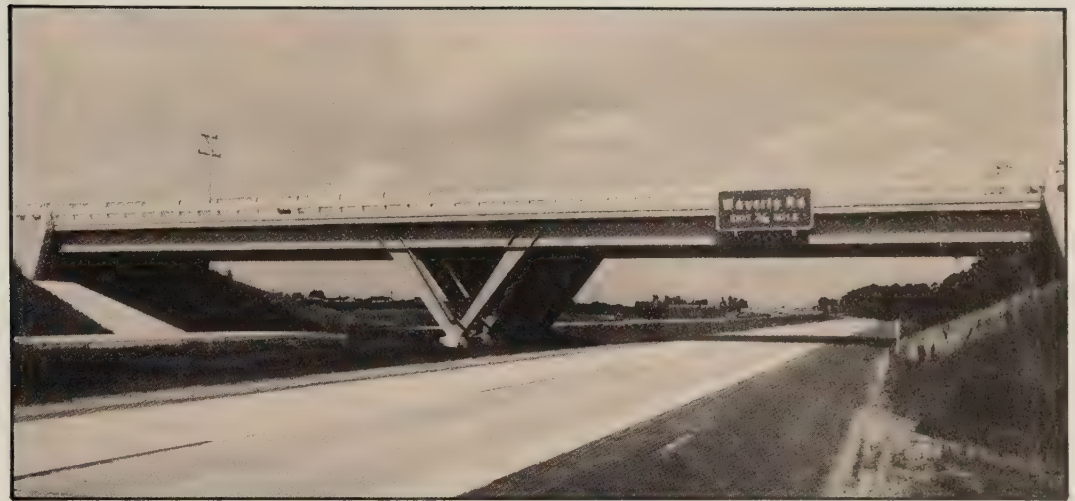
Figure 3. — BRASS may be used to check design calculations and to rate new bridges.
