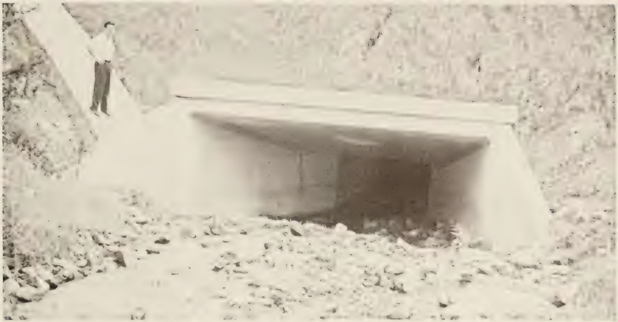
Slope-tapered inlet in North Carolina.
