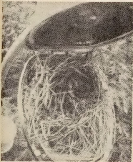
Glassware of this optical assembly has been broken through thermal shock (a condition directly resultant from accumulations of dirt). The fixture has become a haven for birds, rendering the street light totally useless.
