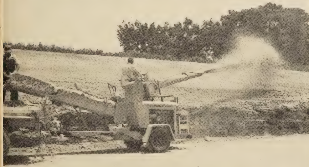
Figure 12.—Mulch blower used to apply hay or straw mulch to slope areas.
