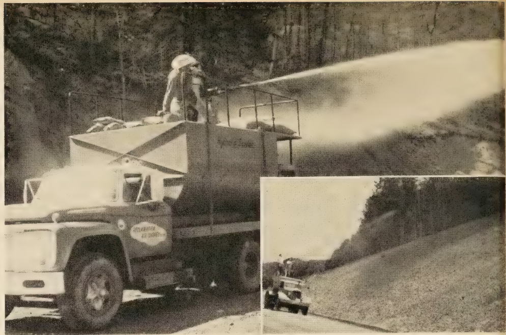
Figure 11.—Hydroseeder used to pump basic ingredients for turf cover on steep slopes.
