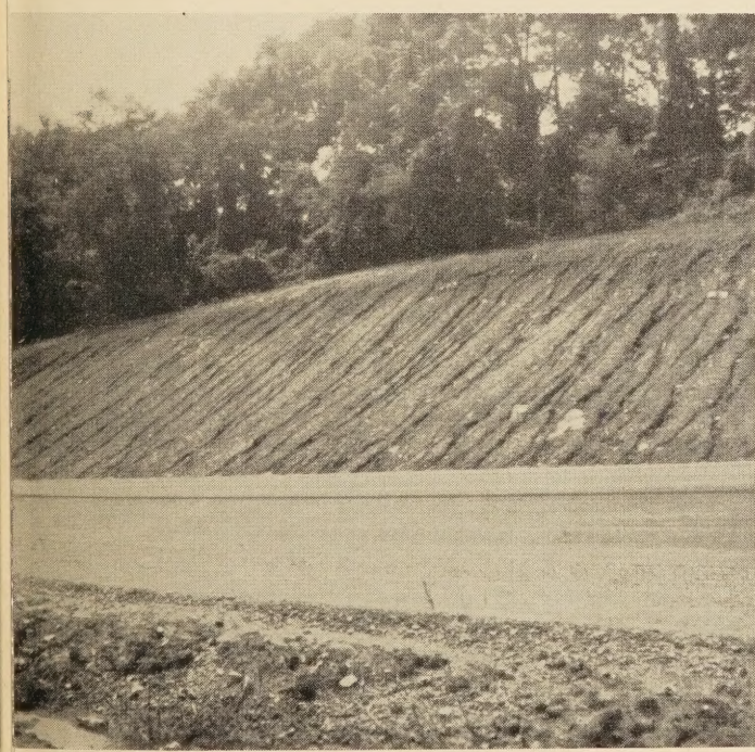
Figure 8.—Erosion and slippage of topsoil can be decreased by proper bonding with slope surface materials.
