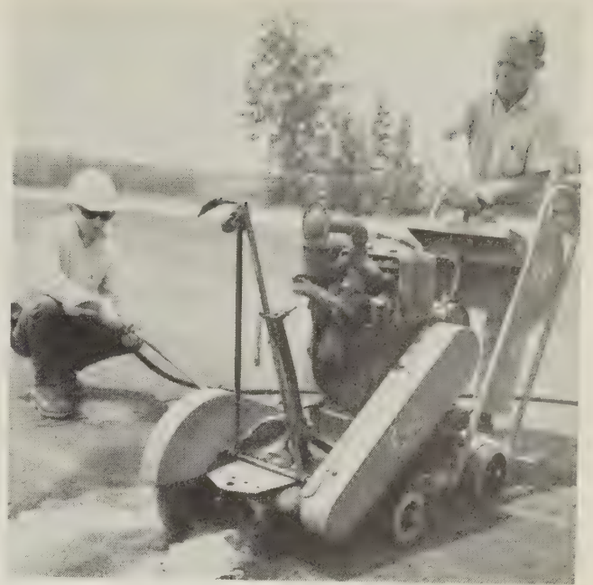
Samples being taken from bituminous pavement for testing— coring a 6-inch diameter sample (left) and sawing a square sample (right).
