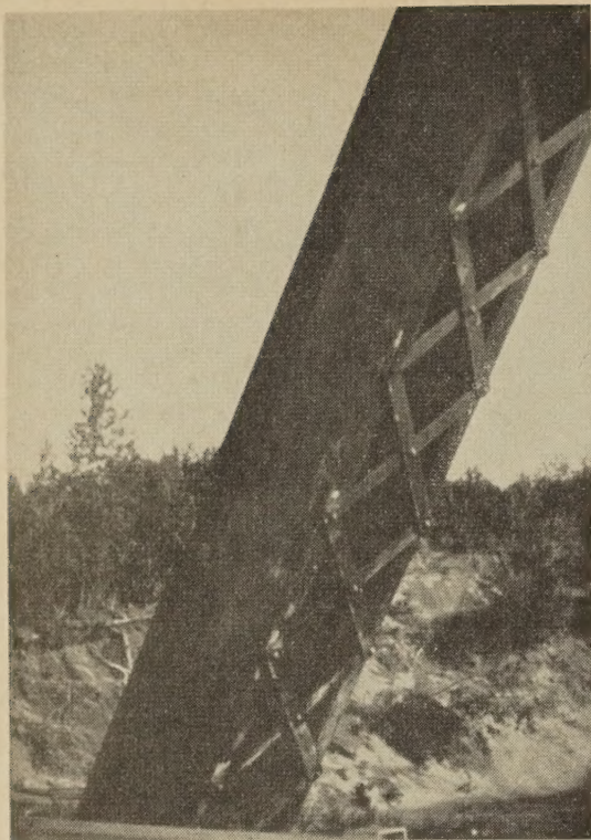
Figure 7.—Paint erosion on end post of Mile 28 Bridge.
