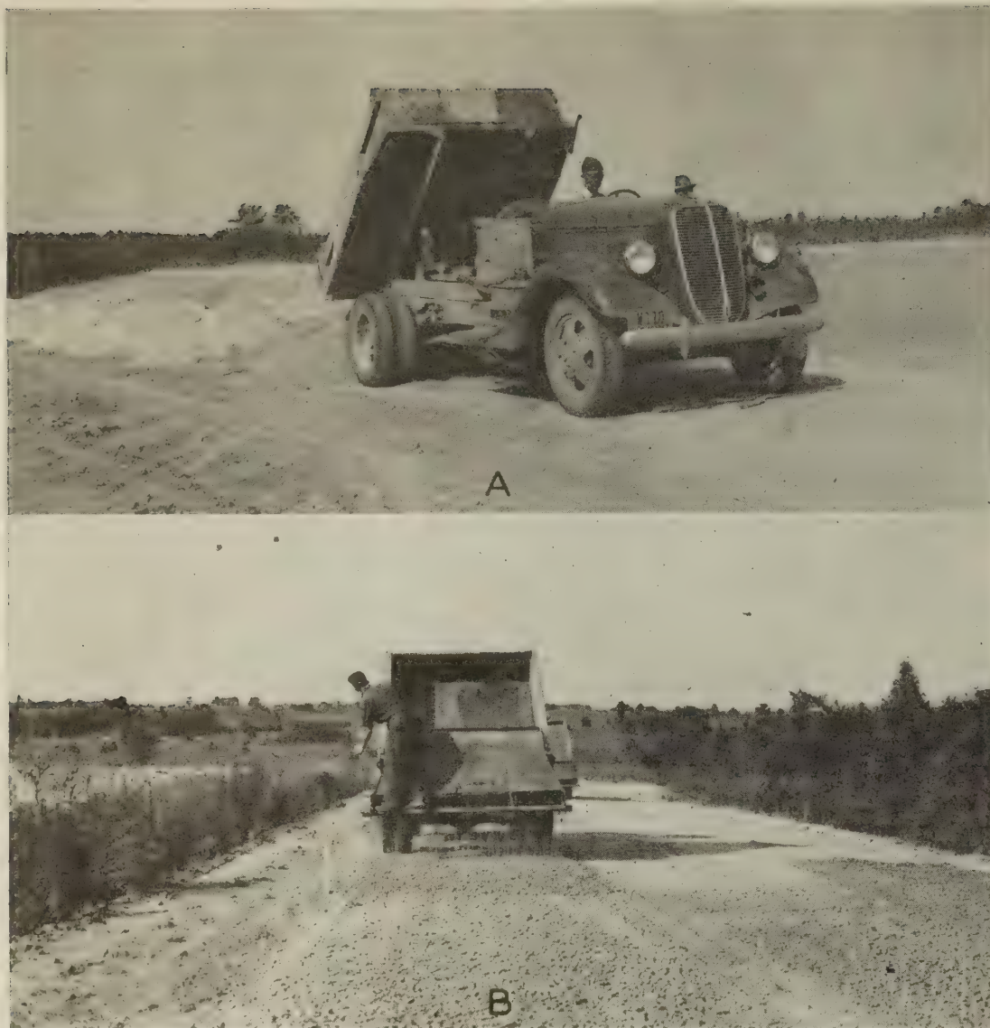
Figure 5.—(A) Placing stone screenings on section 11; (B) spreading crushed stone on section 12.
