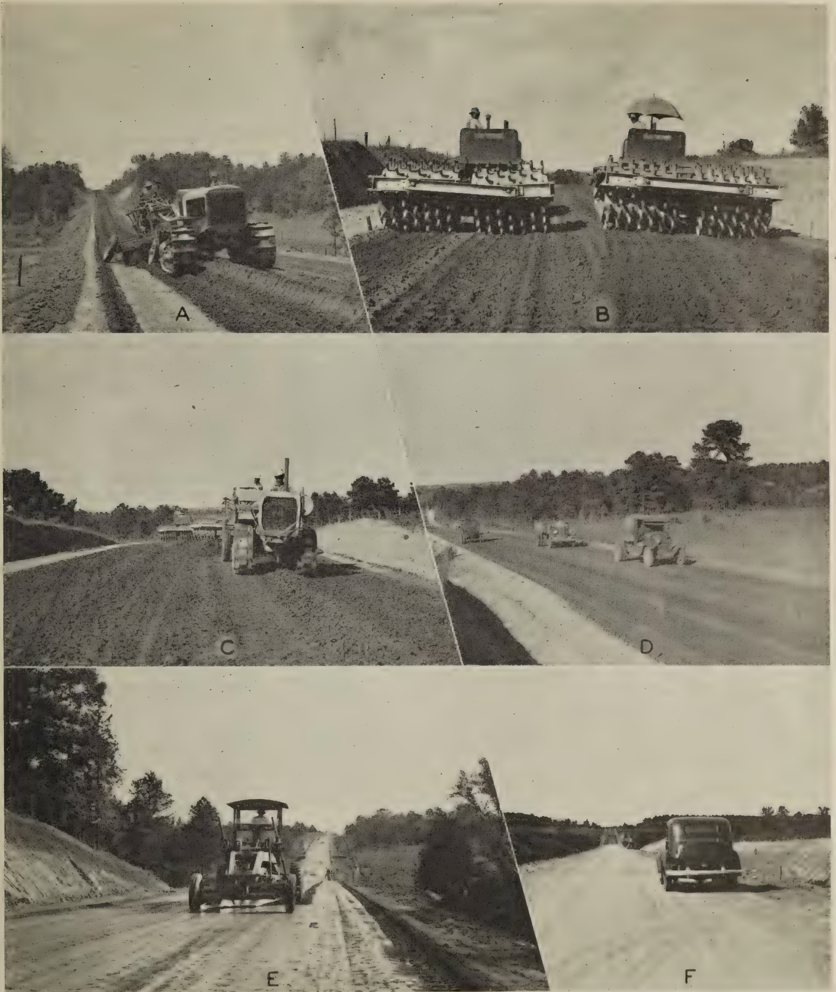
Figure 2.—Soil-cement base-course construction (continued): (A) Wet mixing with a blade grader; (B) compacting; (C) shaping the compacted mixture; (D) rolling with trucks; (E) final blading; and (F) the finished base course.
