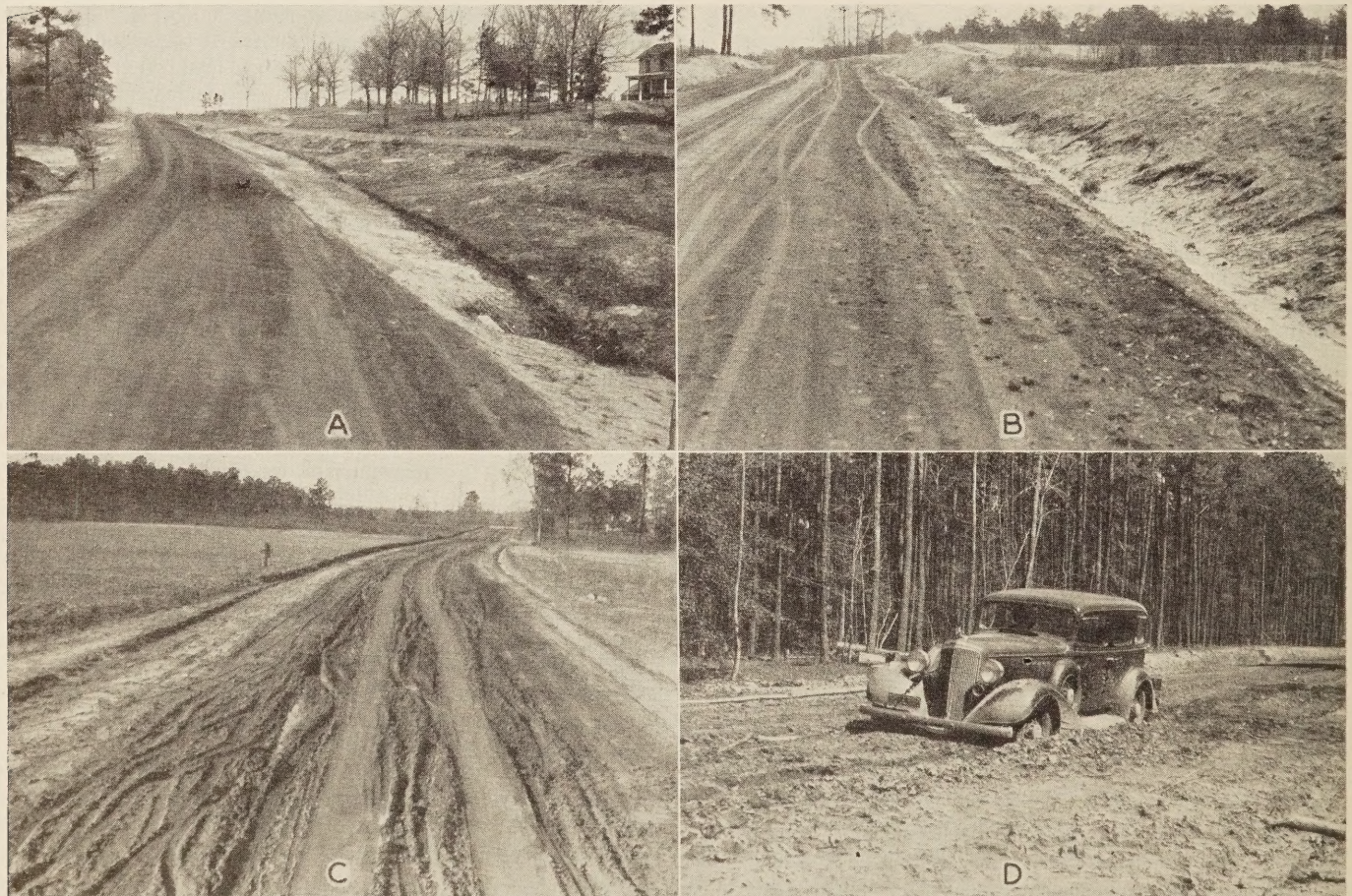
FIGURE 3.—POOR PERFORMANCE OF ORIGINAL SAND-CLAY SURFACING: (A) OUTLET OF POROUS STRATUM CAUSING UNSTABLE AREA; (B) WATER FLOWING FROM SANDY STRATUM IN SIDEHILL CUT; (C) POORLY DRAINED AREA IN PORTSMOUTH SOIL; (D) UNSTABLE ROADWAY IN HIGH WATER TABLE AREA.
