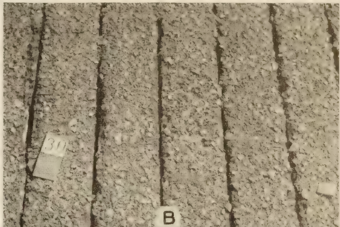
FIGURE 10.—(A) ON A BRIDGE FLOOR WITH LOOSE PLANKS THE FABRIC BROKE QUICKLY. (B) THE CONDITION OF THIS SURFACE ON A SIMILAR BRIDGE IS DUE TO THE EXCELLENT BOND WITH THE PLANKS RATHER THAN THE ABSENCE OF FABRIC.
