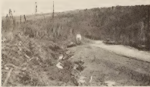
FIGURE 3.—WIDENING THE FAIRBANKS-LIVENGOOD ROAD. REMOVAL OF DENSE COVER OF VEGETATION AND PEAT HAS RESULTED IN DEEPER SUMMER THAWING OF PERENNIALY FROZEN GROUND.
