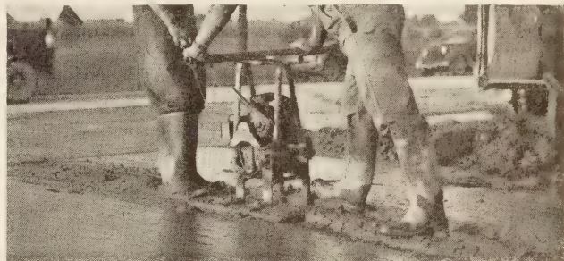
FIGURE 15.—VIBRATORS USED AROUND TYPE III JOINTS. UPPER, VIBRATOR USED ON EAST PROJECT; LOWER, VIBRATOR USED ON WEST PROJECT.
