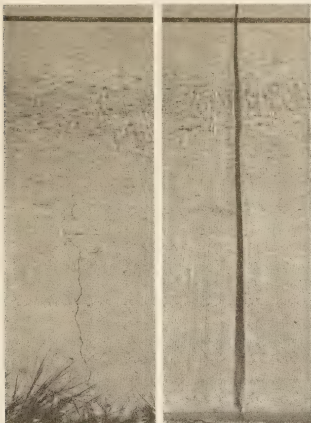
FIGURE 21.—LEFT, CRACK THAT HAS OCCURRED AT A SUBMERGED WEAKENED-PLANE JOINT; RIGHT, WEAKENED-PLANE JOINT WITH SURFACE GROOVE.
