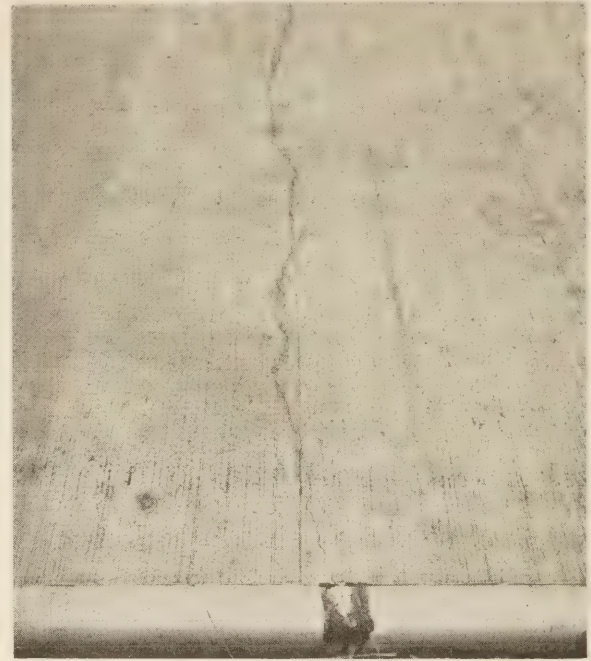
FIGURE 20.—TYPICAL CRACK IN A HEAVILY REINFORCED SECTION.
