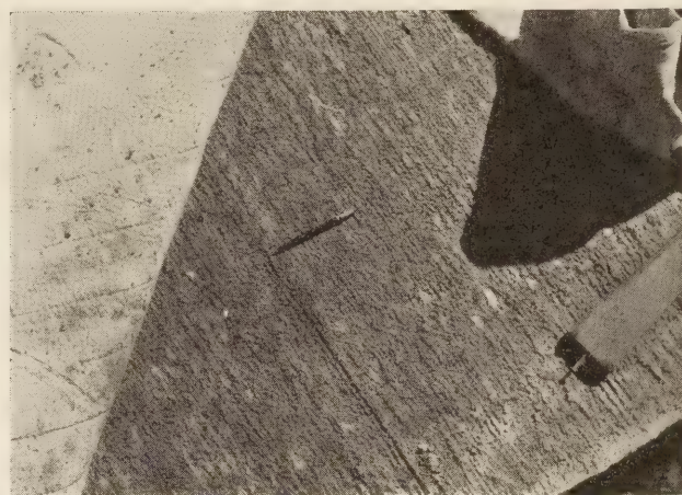
FIGURE 3.—PORTION OF CONCRETE PAVEMENT SLAB AND COTTON MATS USED IN CURING IT.
