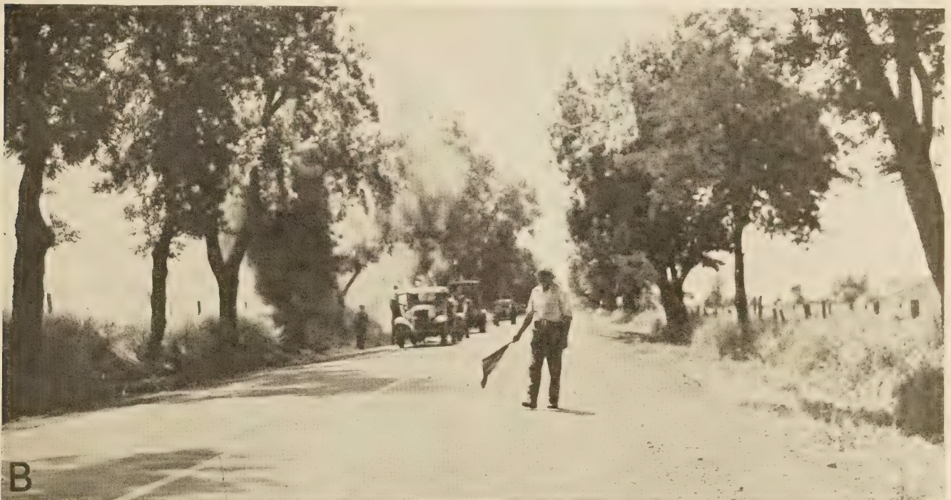
BURNING WEEDS ALONG HIGHWAYS. A, MECHANICAL WEED BURNER; THE INDIVIDUAL OIL BURNERS CAN BE OPERATED SINGLY OR COLLECTIVELY. B, WARNING TRAFFIC OF WEED-BURNING OPERATIONS, WHICH ARE HAZARDOUS TO BOTH TRAFFIC AND DESIRABLE VEGETATION.
