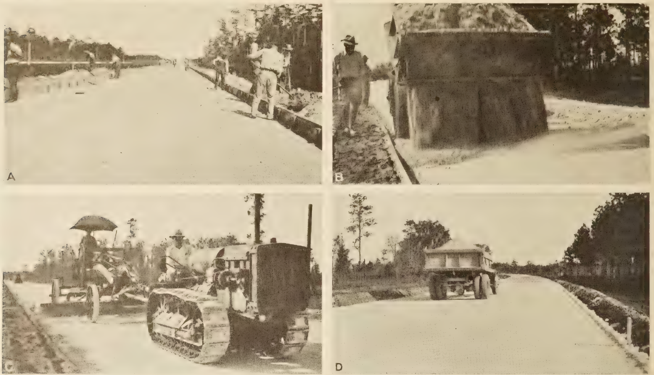
FIGURE 3.—BASE-COURSE ROAD CONSTRUCTION OPERATIONS USING LIMEROCK; A, SUBGRADE PREPARATION. THE SIDE FORMS ARE IN PLACE. B, DUMPING, SPREADING, AND WATERING LIMEROCK; C, BLADING AND FINISHING OPERATIONS; D, FINISHED BASE COURSE READY FOR PRIME COAT.
