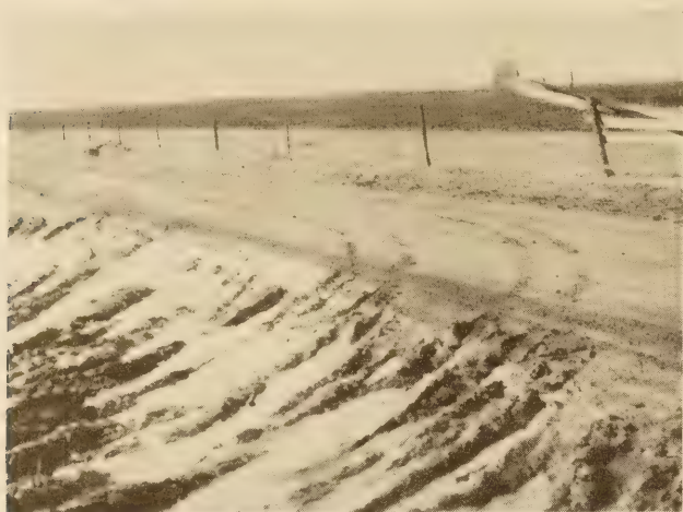
FIGURE 4.—STABILIZED ROAD IN ADAMS COUNTY, PA., AT ITS JUNCTION WITH UNTREATED SIDE ROAD.
