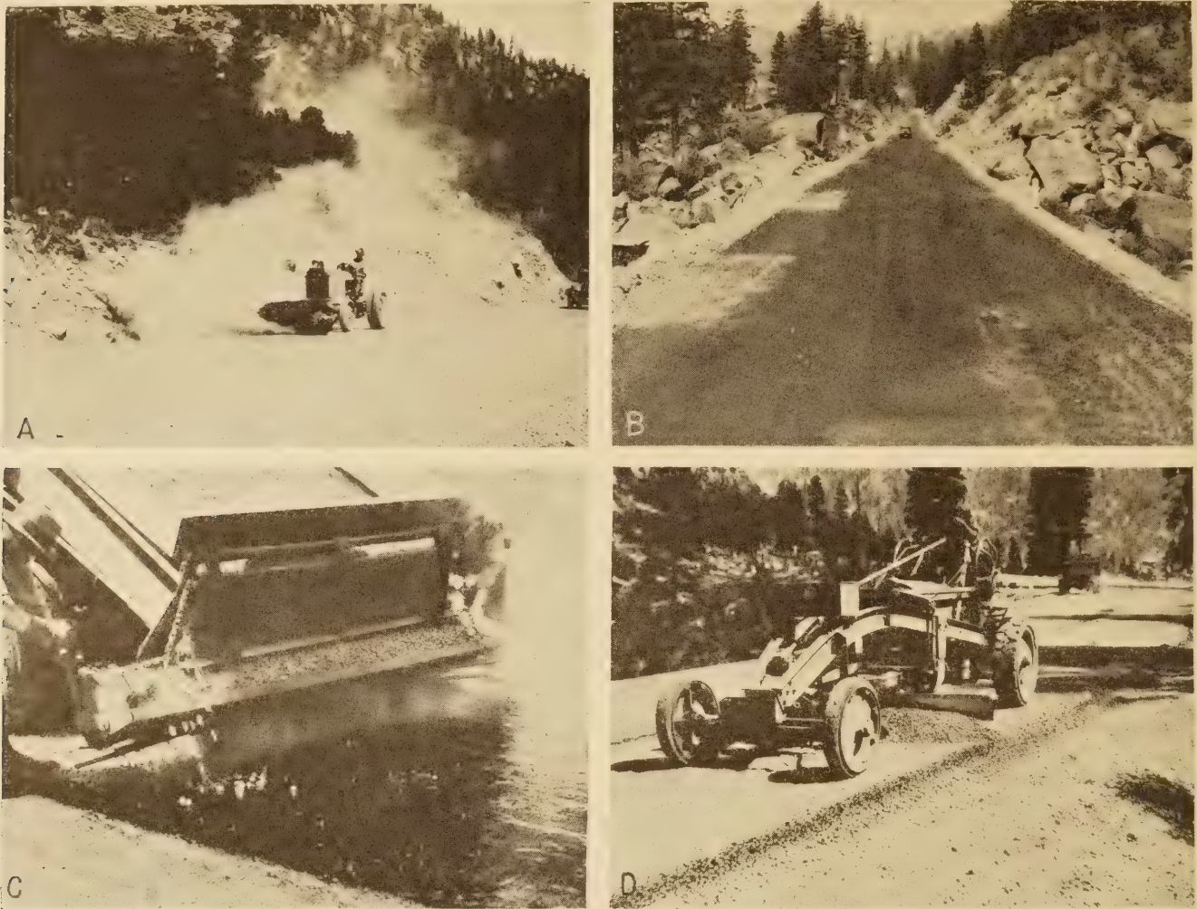
FIGURE 6.—A, SWEEPING BASE BEFORE PRIMING; B, SURFACES PRIMED WITH SLOW-CURING OIL BROKE IN MANY PLACES AND REQUIRED CONSIDERABLE REPAIRING BEFORE APPLYING THE SURFACE TREATMENT; C, SPREADING STONE WITH BOXES ATTACHED TO TRUCKS; D, EQUIPMENT USED TO LIGHTLY MANIPULATE AND SPREAD THE COVER STONE.
