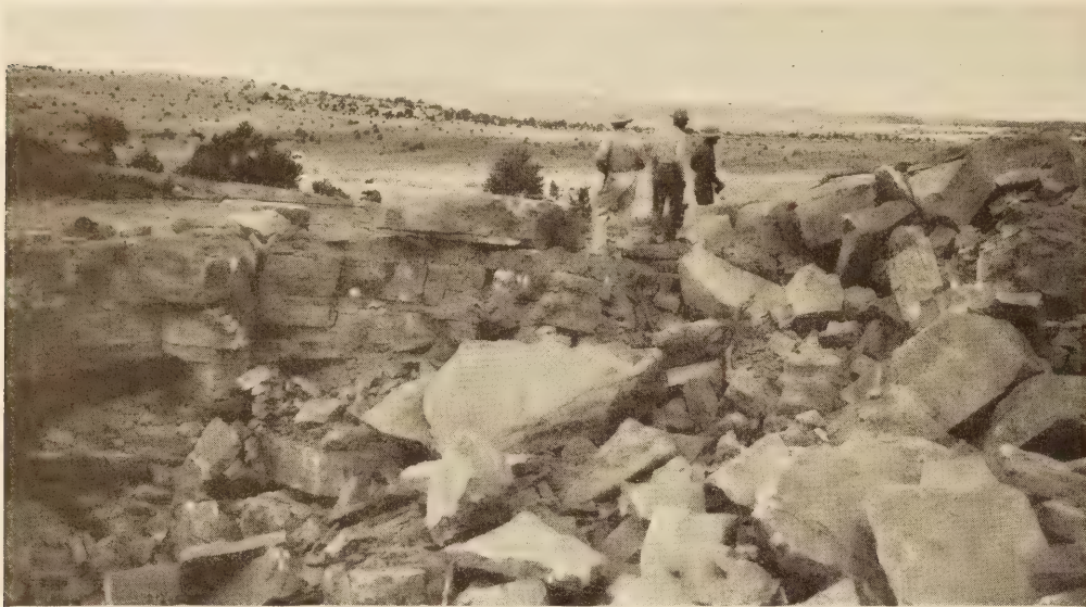
IMPROPER SPACING AND LOADING OF DRILL HOLES RESULTED IN MATERIAL HARD TO LOAD.
