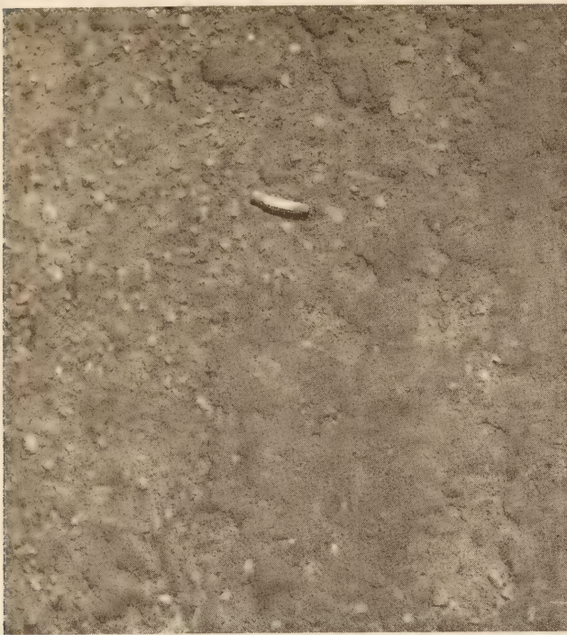
GROUP 3 SURFACE REPRESENTED BY SAMPLE 9. MIXTURE WAS LOW IN OIL CONTENT AND HAD BEEN SEALED TO PREVENT RAVELING. PICTURE SHOWS LOCAL AREA WHERE SEAL HAD PEELED AND RAVELING FOLLOWED. SEALED PORTION REPRESENTED BY SAMPLE 8 WAS IN EXCELLENT CONDITION.
