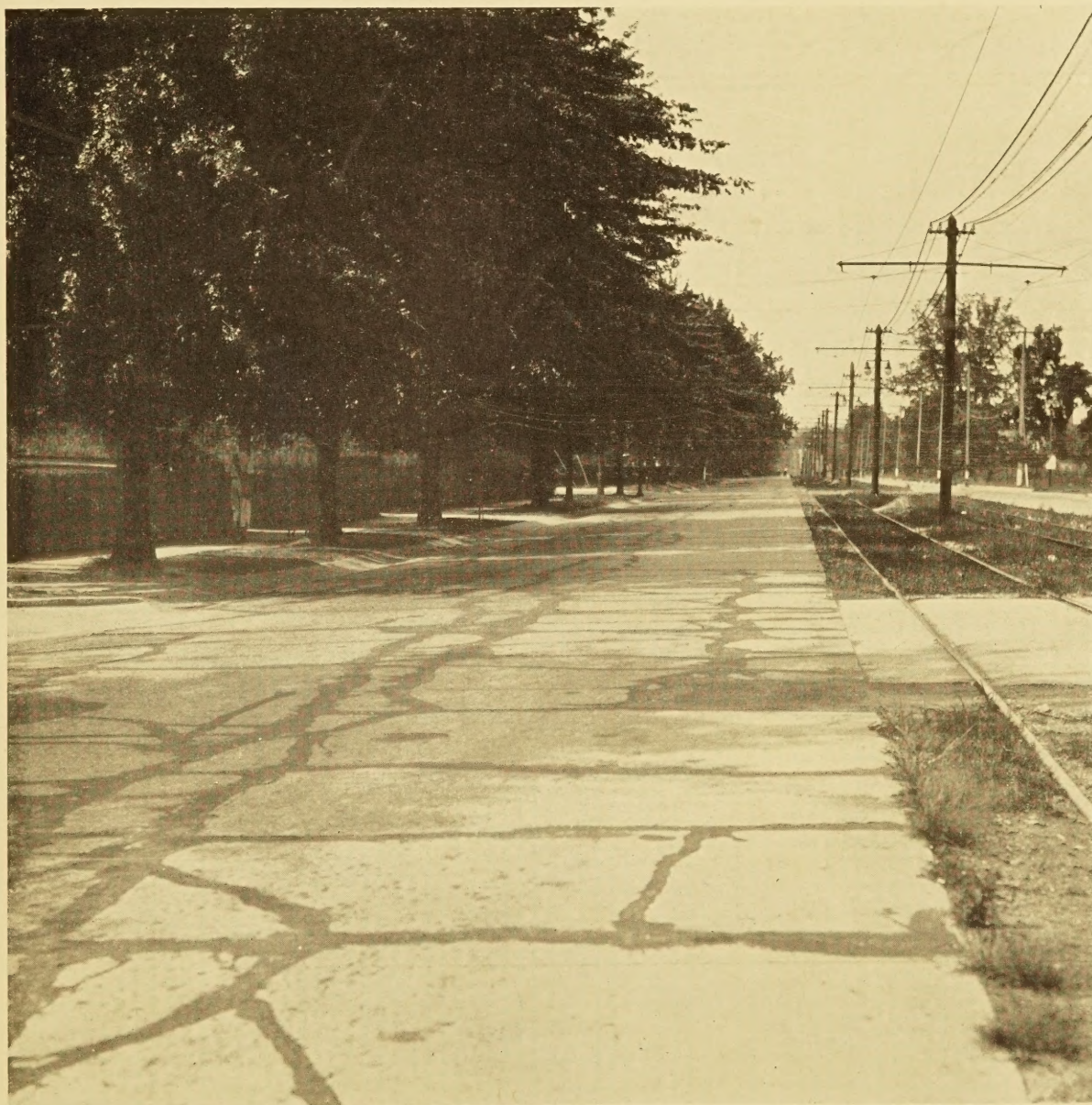
A PORTLAND CEMENT CONCRETE PAVEMENT IN ITS TWENTIETH YEAR
