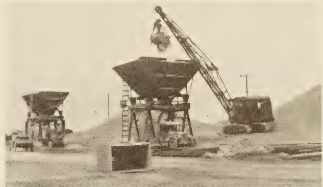
FIGURE 2.—TWO BINS WITH STRAIGHT DRIVE THROUGH BOTH. STOCK PILES ON OPPOSITE SIDES OF TRACK. CRANE WORKING ON A RAMP MADE OF COARSE AGGREGATE
