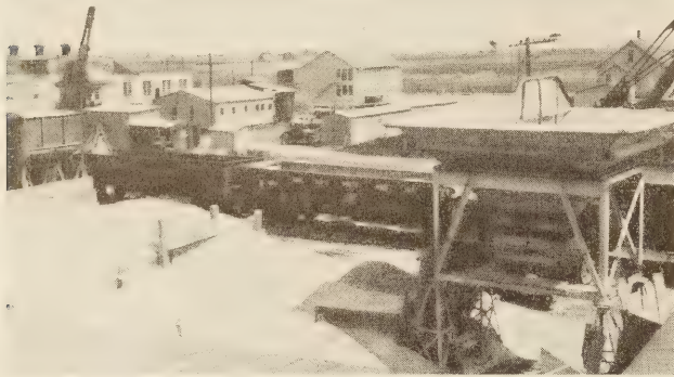
FIGURE 3.—LACK OF ROOM FOR AMPLE STOCK PILES AND SPECIFICATIONS REQUIRING THREE SIZES OF COARSE AGGREGATE NECESSITATED THE USE OF TWO CRANES
