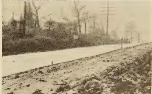
FIGURE 5.—WARPED SLABS. TRANSVERSE JOINTS ARE MARKED WITH STICKS
