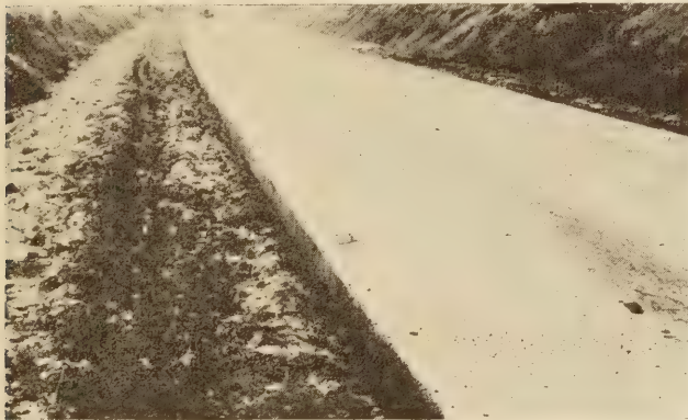
FIGURE 4.—SHOULDERS ARE RUTTED TO A DEPTH OF 4 INCHES BELOW BOTTOM OF SLAB
