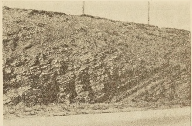
FIGURE 5.—STRATIFICATIONS IN SHALE. THE CONTACT PLANES BETWEEN THE DIFFERENT SHALE STRATA ARE POTENTIAL PLANES OF WATER SEEPAGE
