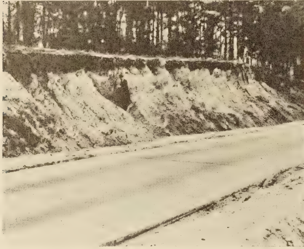
FIGURE 2.—EROSION OF BACK SLOPES IS VERY IRREGULAR AND THERE IS CONSIDERABLE SLOUGHING OF MATERIAL INTO DITCHES
