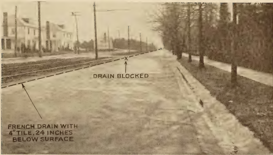
FIGURE 4.—SECTION 3, NORTH OF BRADLEY LANE, FEBRUARY, 1929. APPEARANCE OF SECTION JUST NORTH OF VIRGILIA STREET. SHINY AREAS ARE WATER WHICH HAS COME UP THROUGH THE CRACKS IN THE CONCRETE PAVEMENT. NOTE WATER WHICH HAS FLOWED FROM THE SURFACE INTO THE GUTTER AT THE RIGHT
