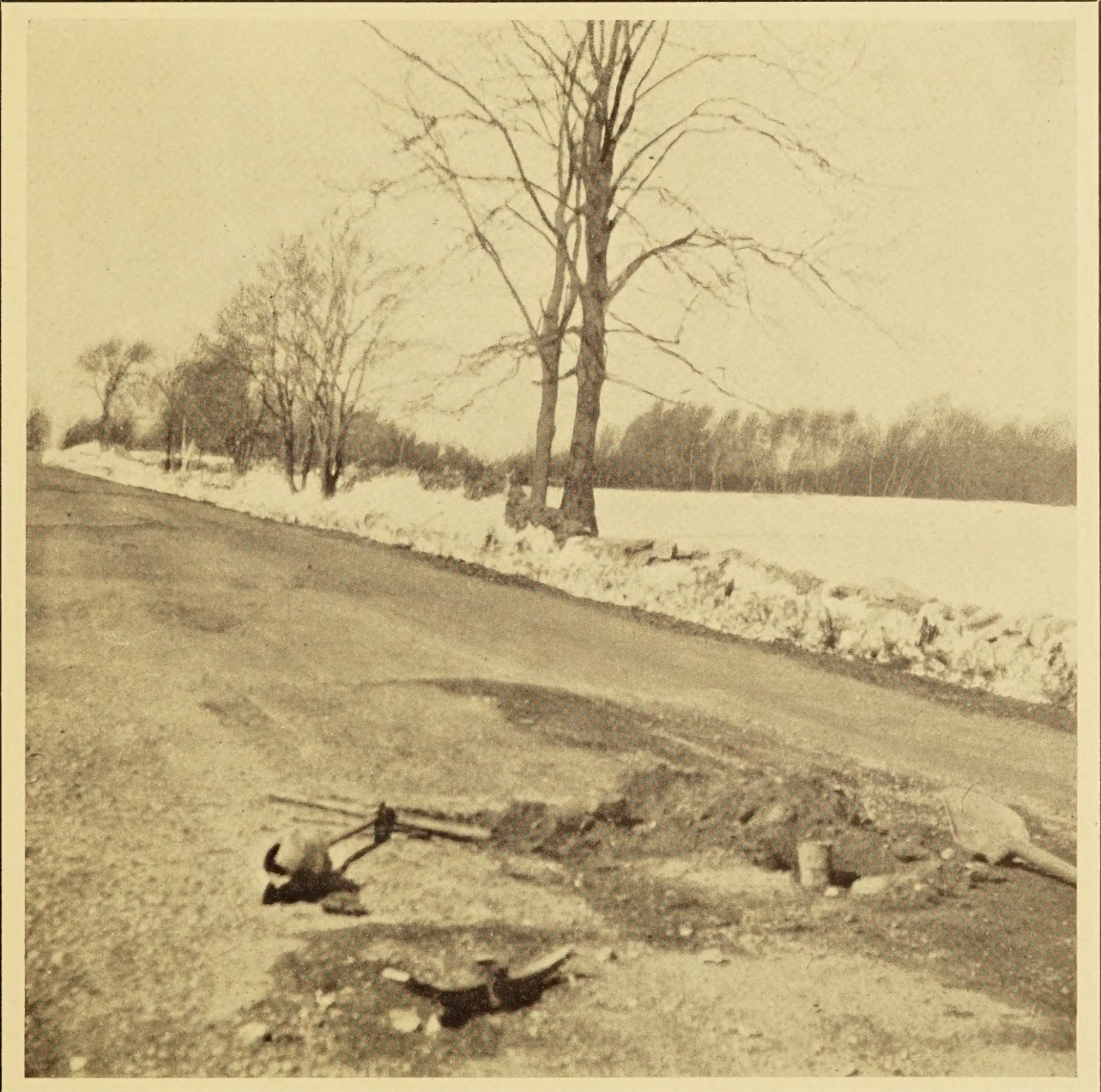
HIGHWAY DAMAGED BY GROUND FREEZING
