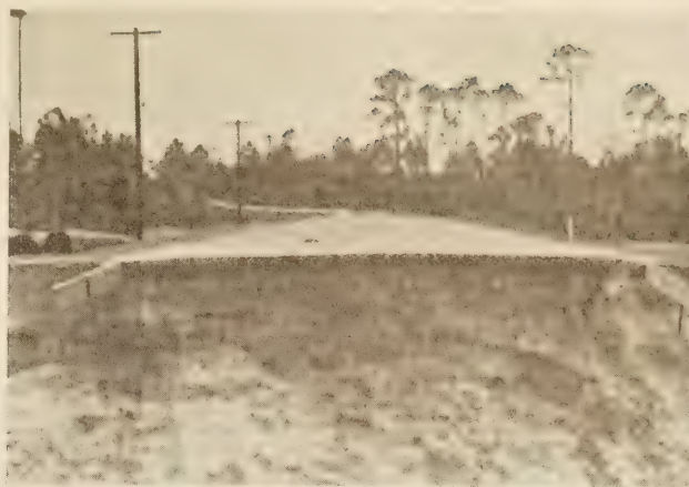
CROSS SECTION OF SURFACE TREATED SAND-CLAY ROAD (RESULT OF WASHOUT) SHOWING SUBSOIL AND WOODEN CURBS. SECTION 1 IN FLORIDA
