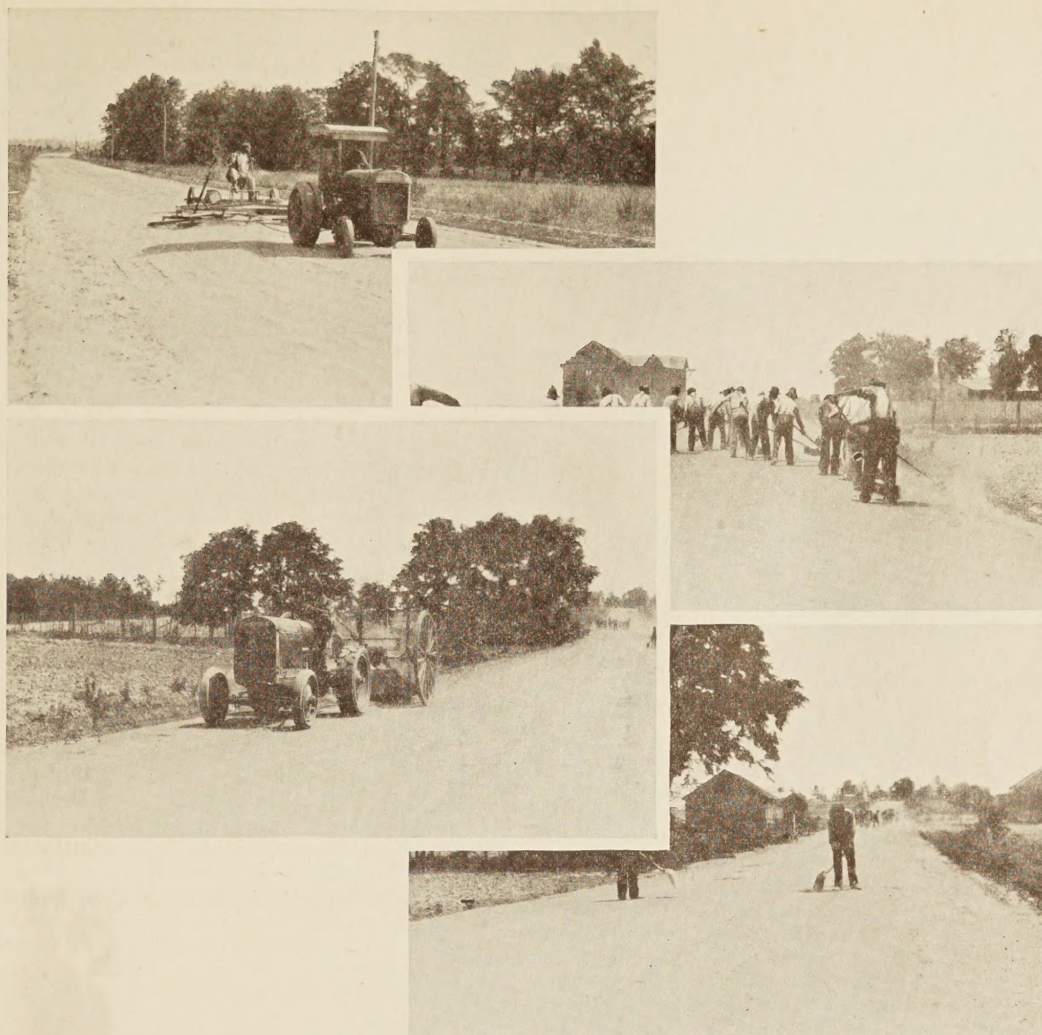
STEPS IN PREPARING A SAND-CLAY SURFACE FOR SURFACE TREATMENT. NOTE THE V-FORMATION OF SWEEPERS
