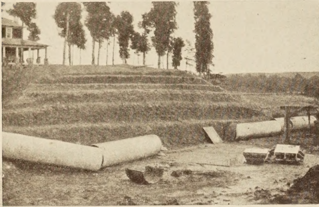
FIGURE 12.—FILL STEPPED BACK TO PREVENT ARCH ACTION OF THE SOIL OVER PIPE
