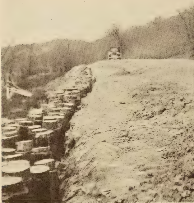
CLOSELY SPACED PILING TO HOLD A ROAD IN PLACE USE OF WOOD PILES HAS DISADVANTAGES
