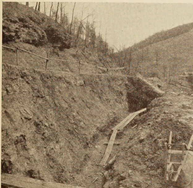
EXCAVATION FOR RETAINING WALL TO HOLD ROAD SHOULDER, NEAR WEST UNION, W. VA.
