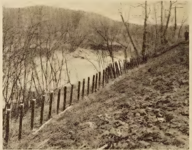
CASING FILLED WITH REINFORCED CONCRETE USED TO RETAIN A FILL. OAK PILING NEARER THE RIVER HAS FAILED AND THE CONCRETE PILING IS BEGINNING TO FAIL. DRAINAGE OF A SWAMPY AREA ON THE OTHER SIDE OF THE ROAD APPEARS TO BE THE REMEDY
