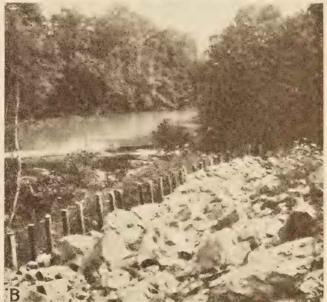
MASSSES OF ROCK PLACED AT TOE OF SLIDING FILL TO SUPPLEMENT PILING
