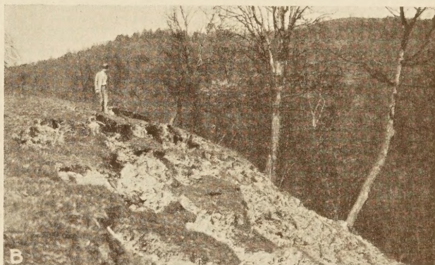
A SLIDE IN PUTNAM COUNTY, W. VA., WHICH OVERTURNED A RETAINING WALL
