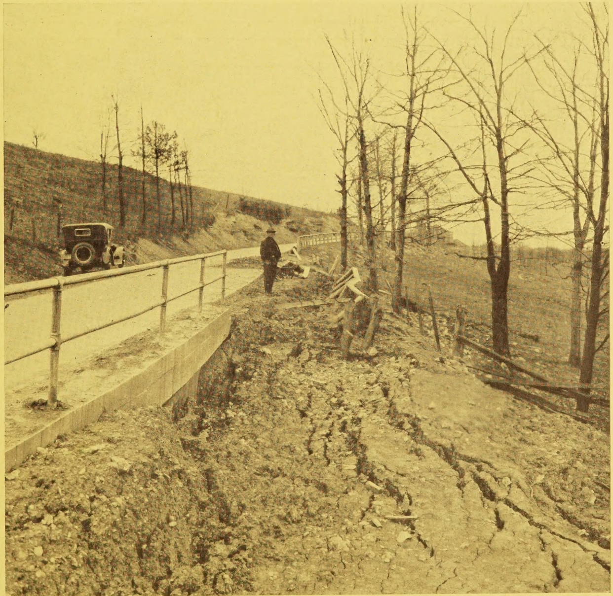
A TYPICAL LANDSLIDE IN WEST VIRGINIA
