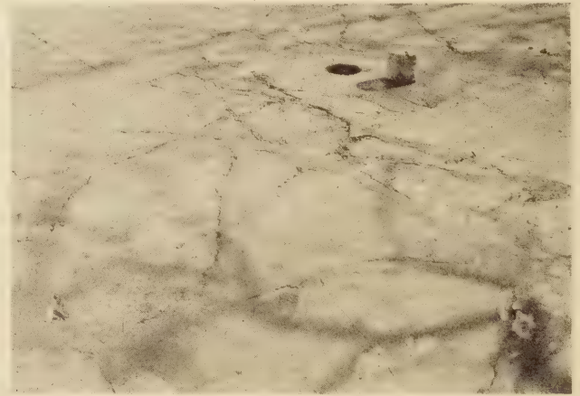
BADLY CRACKED CONCRETE PAVEMENT IN 1928 WHICH PRODUCED CORES OF FAIRLY HIGH STRENGTH
