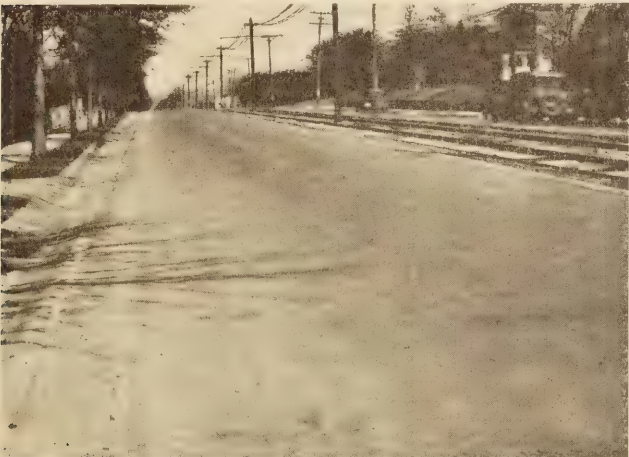
CONDITION OF BITUMINOUS CONCRETE SECTIONS IN 1928. THE THE UPPER PICTURES ARE OF EXPERIMENT 1 AND THE LOWER IS OF EXPERIMENT 2
