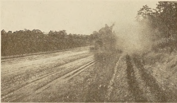
FIRST APPLICATION OF BITUMINOUS MATERIAL TO A PORTION OF THE SOIL. SECOND APPLICATION TO FOLLOW AFTER SPREADING THE SOIL SHOWN IN WINDROWS
