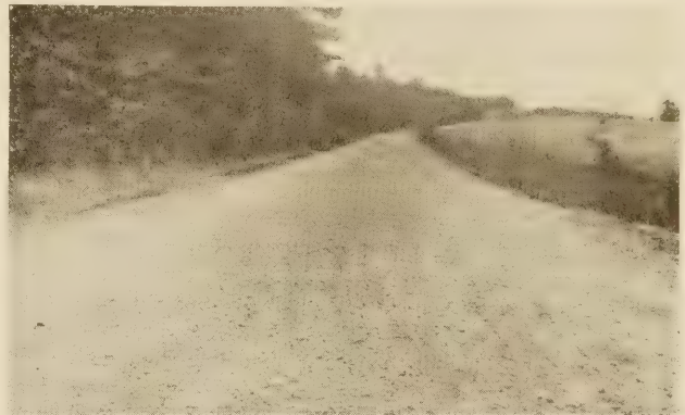
APPEARANCE OF DOUBLE SURFACE TREATMENT SHORTLY AFTER CONSTRUCTION. PATROL MAINTENANCE NEEDED AT THIS STAGE TO RESPREAD LOOSE COVERING AND REPAIR BROKEN PLACES
