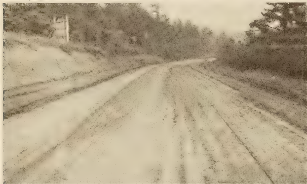
A TOPSOIL SURFACE LOOSELY BONDED AND NOT SUITABLE FOR DOUBLE SURFACE TREATMENT. A SLOW-DRYING OIL PENETRATION OR MIXED TREATMENT WOULD BE BETTER FOR THIS CONDITION
