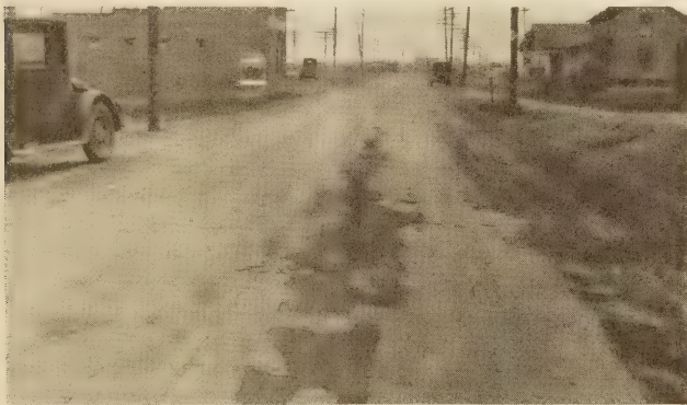
AN EXAMPLE OF EXCESSIVE SCALING DUE TO THE IMPROPER SELECTION OF SURFACE TREATMENT MATERIALS
