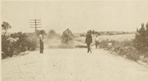
STONE COVERING APPLIED IMMEDIATELY AFTER THE APPLICATION OF THE HOT TOP COAT
