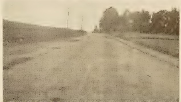
TAR PENETRATION TREATMENT ON SECTIONS 3 AND 4. THE THIN BRITTLE SURFACE BROKE AND SCALED BADLY DURING THE FIRST YEAR BUT WAS MATERIALLY STRENGTHENED BY LATER RE-TREATMENTS
