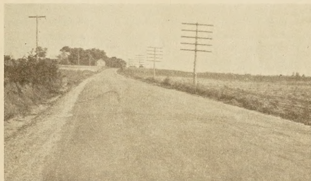
A DOUBLE SURFACE TREATMENT AFTER TWO YEARS SERVICE
