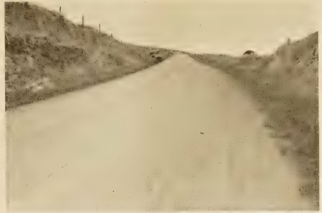
FIG. 19.—MILE 226 ON COLUMBIA RIVER HIGHWAY. RE-SURFACED AND TREATED WITH OIL AT A RATE OF 0.24 GALLON PER SQUARE YARD IN 1923 AND AN ADDITIONAL TREATMENT OF 0.26 GALLON PER SQUARE YARD IN 1924
