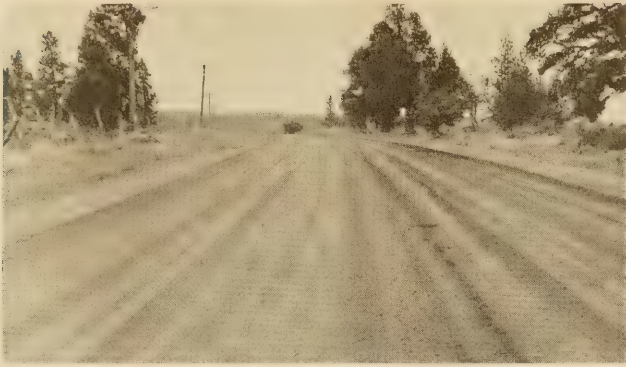
FIG. 21.—CONDITION OF OILED SURFACE ON MILE 130 OF THE DALLES-CALIFORNIA HIGHWAY IN AUGUST, 1926
