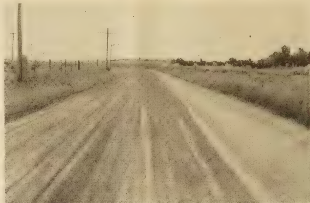
FIG. 16.—MILE 196 ON COLUMBIA RIVER HIGHWAY. RESURFACED IN 1924. OIL APPLIED AT A RATE OF 0.495 GALLON PER SQUARE YARD IN 1925. SURFACE RECENTLY REOILED LIGHTLY AND SANDED
