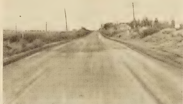
FIG. 13.—MILE 185 OF COLUMBIA RIVER HIGHWAY. RE-SURFACED IN 1923 AND OILED IN 1925. THE SURFACE BECAME BADLY RUTTED AND IN APRIL, 1926, A TAR TREATMENT WAS APPLIED WITHOUT APPARENT BENEFIT. A SURFACE SAMPLE SHOWED AN EXCESS OF CLAY SATURATED WITH MOISTURE
