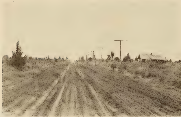
FIG. 22.—MILE 115.8 ON THE DALLES-CALIFORNIA HIGHWAY SHOWING SURFACE BROKEN UP. A SECTION CAN BE SEEN IN THE DISTANCE WHERE ONLY THE EDGES ARE BROKEN
