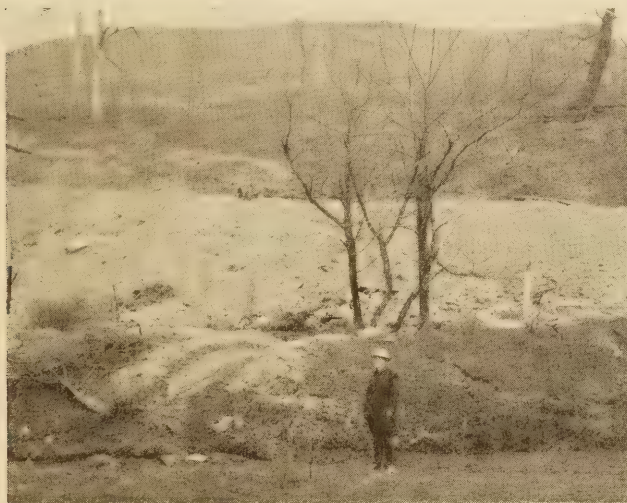
FIG. 24.—UPHEAVAL OF OLD DETRITUS CAUSED BY WEIGHT OF FILL. NEW CRACKS CAN BE SEEN AT BACK OF MAN. THE STABILITY OF THE ROAD UNDER SUCH CONDITIONS IS EXTREMELY UNCERTAIN
