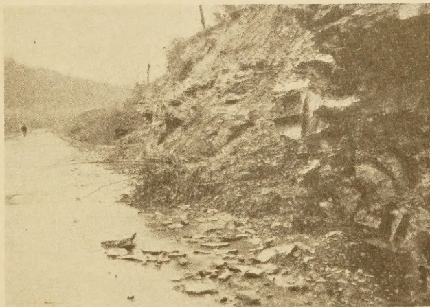
FIG. 2.—IN SOME LOCATIONS THERE IS A CONTINUOUS FALL OF MATERIAL UPON THE HIGHWAY AND IT IS PARTICULARLY HEAVY IN THE WINTER AND SPRING MONTHS
