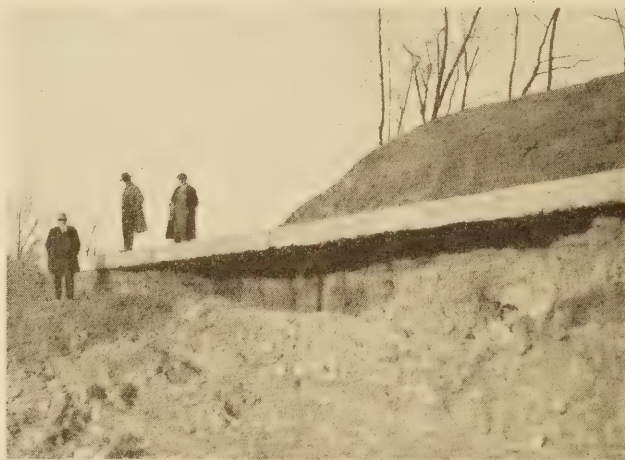
FIG. 22.—A FILL SLIDE THAT HAS UNDERMINED A CONCRETE ROAD. OFTEN LARGE SECTIONS OF THE ROAD BREAK OUT AND ARE CARRIED AWAY
