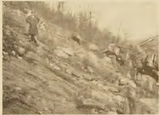
FIG. 18.—VIEWS LOOKING UP AND ACROSS A 45° SLOPE WHERE A SLIDE OF STRATIFIED ROCK OCCURRED AS A RESULT OF A HIGHWAY CUT
