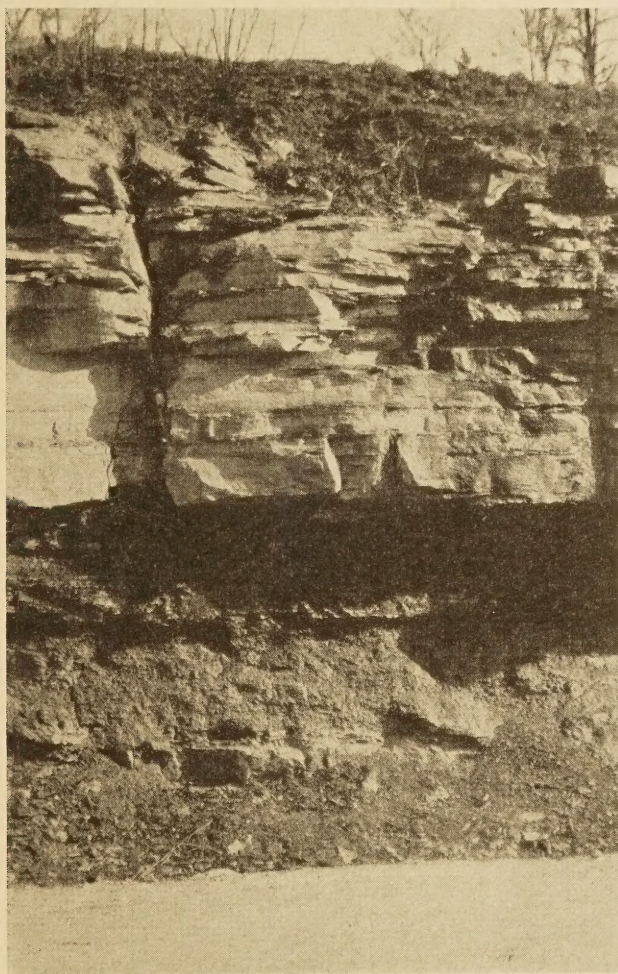
FIG. 6.—BED OF SANDSTONE BEING UNDERMINED BY WEATHERING OF UNDERLYING SHALE. NOTE THE VERTICAL JOINT IN THE SANDSTONE
