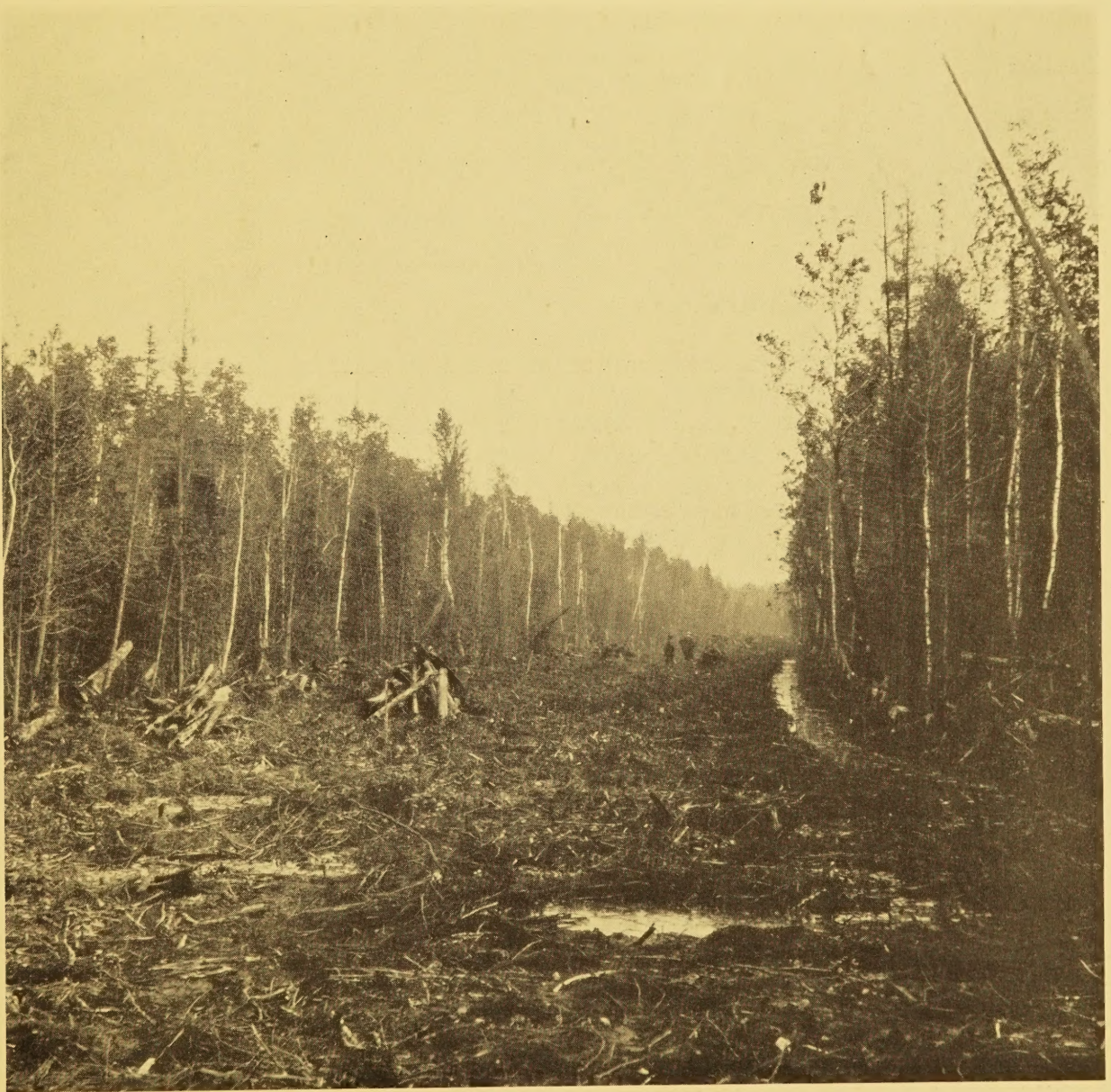
ROAD CONSTRUCTION OVER PEAT BOGS HAS PRESENTED A DIFFICULT PROBLEM IN MICHIGAN
