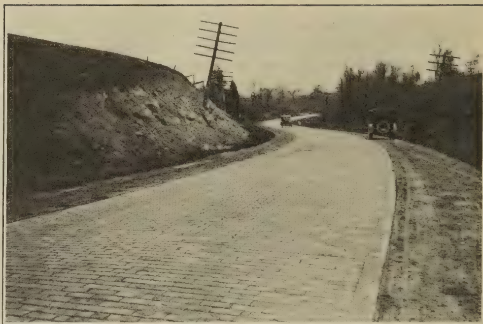
FIG. 3.—REPRESENTATIVE SECTION OF THE NATIONAL ROAD, A TAR-MASTIC FILLED BRICK ROAD ON A CRUSHED SANDSTONE BASE.
