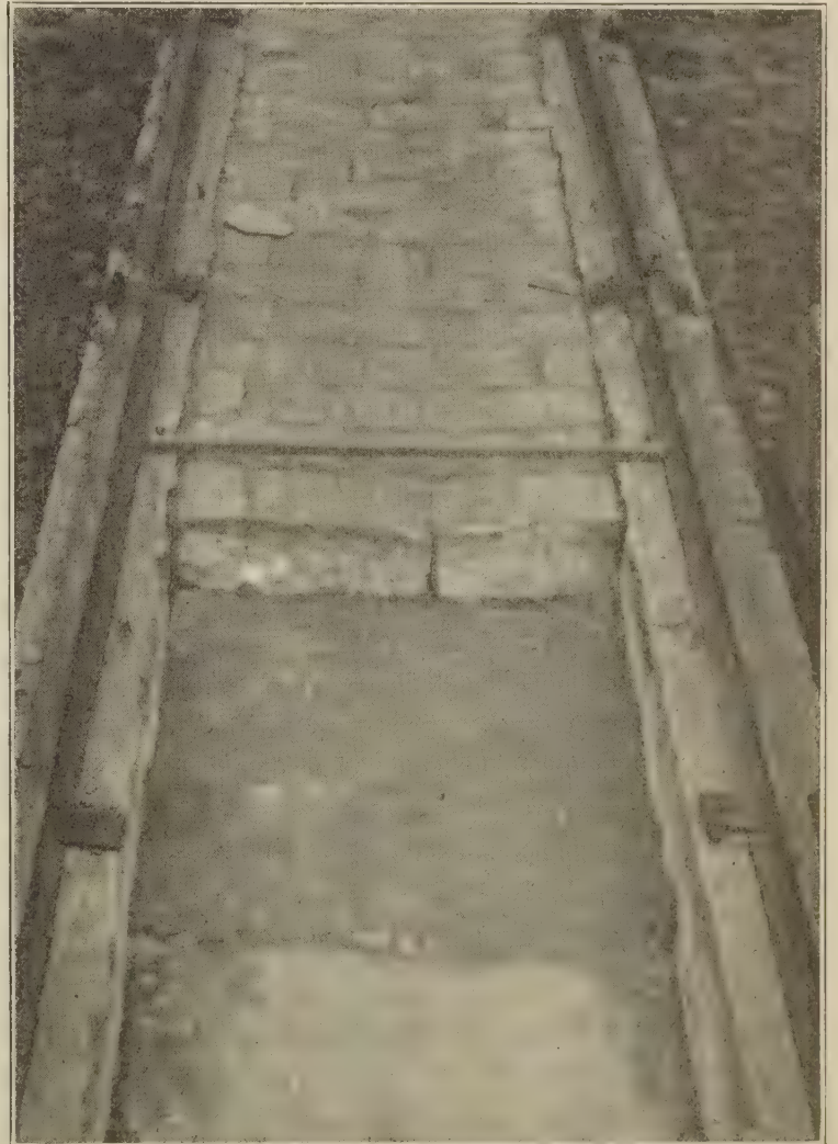
DETAILED VIEW OF SECTION 1, SHOWING SETTLEMENT AND PINCHING ACTION ON UPPER EDGE OF BLOCK.
