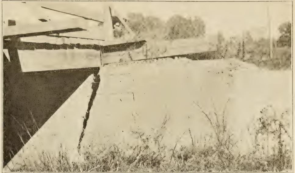
FAILURE OF AN ABUTMENT SUPPORTING A WOODEN SUPERSTRUCTURE. INSUFFICIENTLY DESIGNED ABUTMENT. FAILURE RESULTED PRIMARILY FROM SCOURING OF FOUNDATION.
