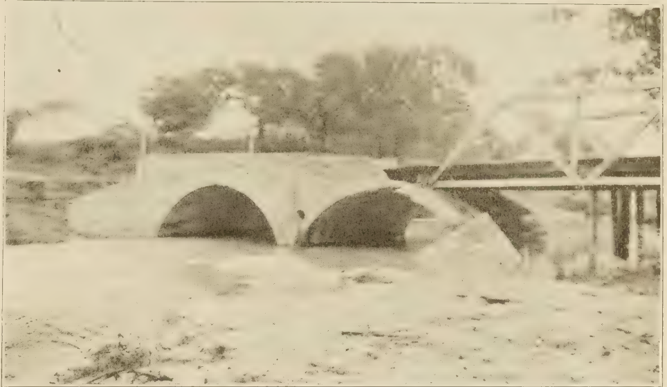
REINFORCED CONCRETE ARCH BRIDGE WRECKED BY STREAM SCOUR. AS CONSTRUCTED, BRIDGE HAD SHALLOW FOUNDATION ON GRAVEL. WATERWAY APPROXIMATELY 50 PER CENT THAT REQUIRED.
