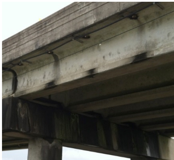
Figure 5: Outside edge of bridge showing concave configuration which traps an air pocket when a wave strikes it and potentially increases lateral loads.
