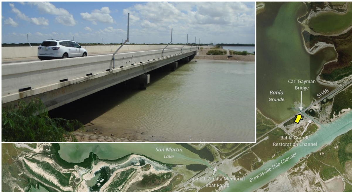
Figure 8. South Side View of the Carl Gayman Bridge along SH 48 Showing Pelican Poles and the Relatively Low Height from the Tidal Water Surface to the Bottom of the Bridge Deck Structure. The CTB-mounted pelican poles are visible on the side of the bridge. The yellow arrow on the map indicates approximate photo location and direction.
