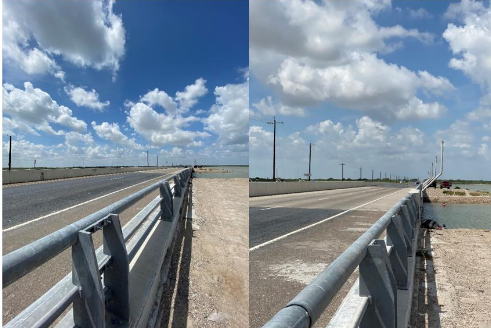
Figure 11. View of New Guard Rails Installed on the Carl Gayman Bridge. View to the southwest along westbound SH 48. Left image shows the space between each horizontal crossbar on the railing. The right image shows the reinstated pelican poles and a new transmission line on the south side of the highway (image captured January 2021).
