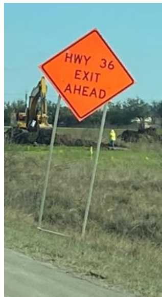
(a) Advance guide sign
