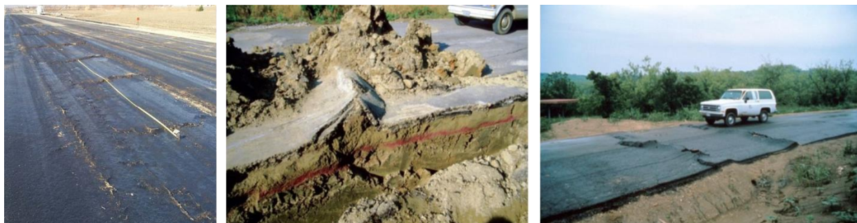
Figure 2: Examples of Damaging Effects of Expansive Soils on Pavements. 12
