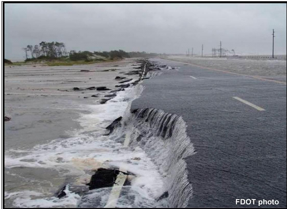
Figure 3: Photograph of the weir-flow damage mechanism occurring in 2005 on the stretch of US 98 selected for this assessment. This photograph was taken looking toward the east during a small tropical storm (after the highway had been repaired from Hurricane Ivan damage). This is the north edge of pavement on the westbound lanes. Note that the damage is on the side of the roadway away from the ocean! Choctawhatchee Bay is to the left and the Gulf of Mexico is to the right. The flow is south to north (right to left) during the incoming storm surge. 14
