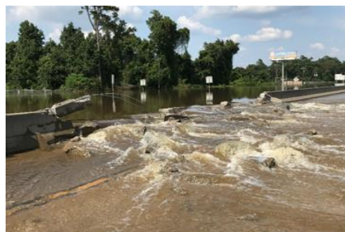
(a) In Beaumont, Texas, several sections of median barrier were exploded to help mitigate the increased flooding being caused by the solid concrete barrier (2).
