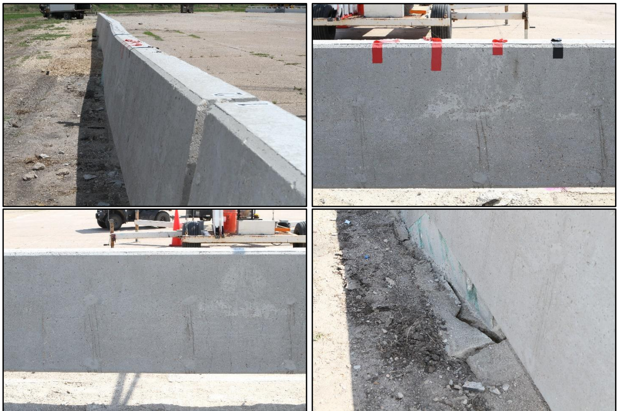
Figure 11.5. Field Side of Barrier after Test No. 469760-06-3.
