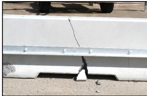
Figure 2.20. Concrete Crack after MASH Test 3-11 (Retrofit System).
