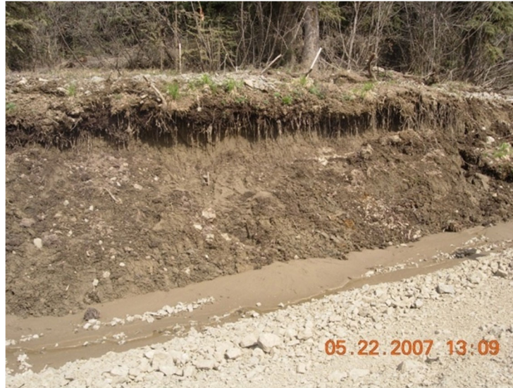
Figure 6-4 Advanced cut slope thaw with silty runoff flowing in ditch and general slumping of coarse material.
