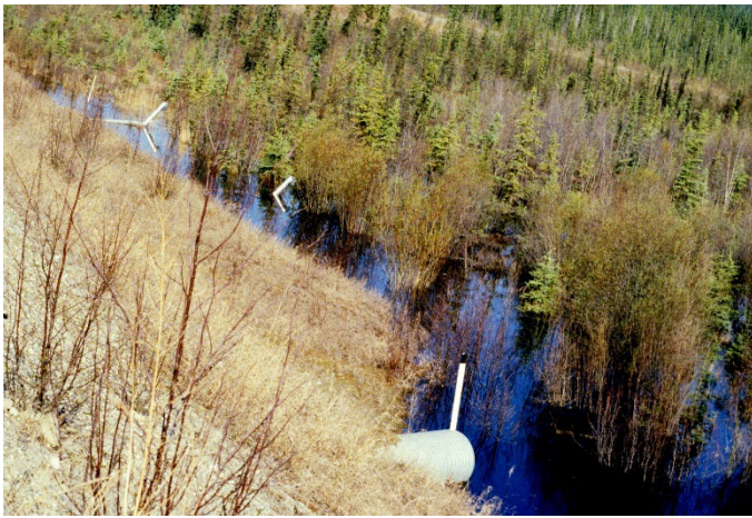
Figure 7-5 Water ponding in Talik formed at toe of slope.
