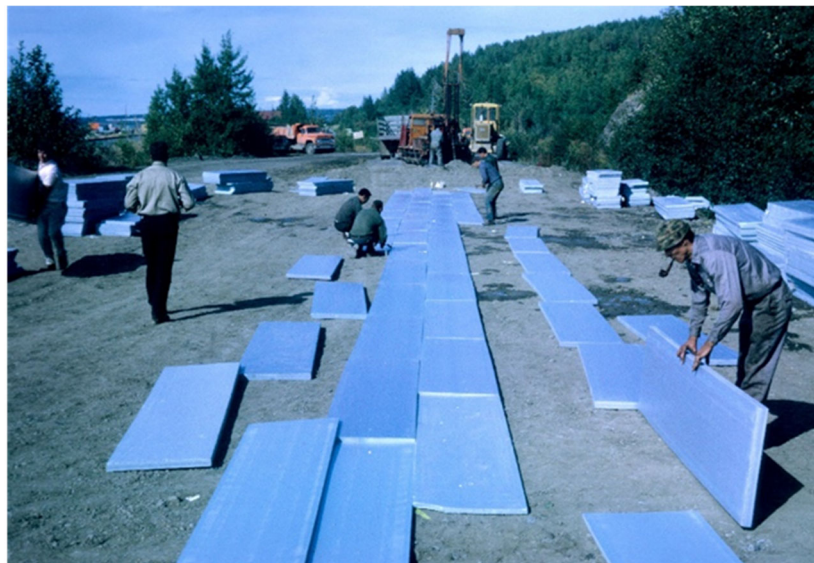
Figure 5-4 Installation of DOW Extruded Foam Insulation at Fairhill Road near Fairbanks, AK
