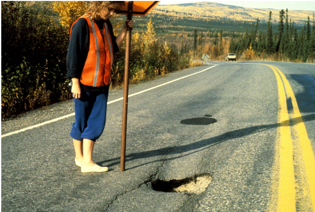
Figure 5-1 Roadway damage resulting from thawing permafrost. Photo by Thomas Kinney
