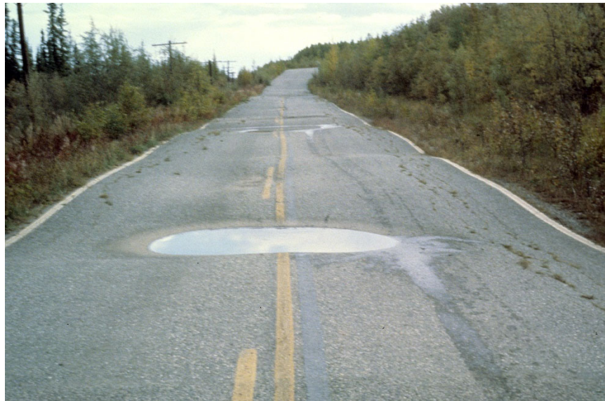
Figure 1-3 Roadway damage on an abandoned section of the Richardson Highway east of Fairbanks (photo B. Connor)
