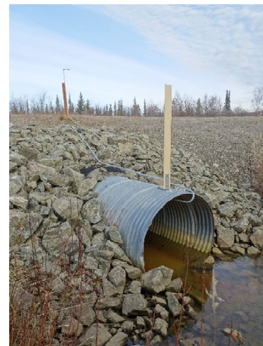
Figure 7-13 Use of Riprap to reduce slope damage due to thaw settlement.
