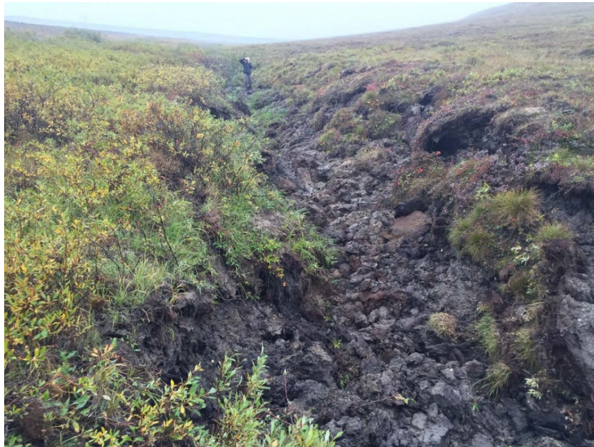
Figure 7-3 Erosion due to Advection due to installation of fiber optic cable along the Dalton Highway. Photo by Mikhail Kanevskiy
