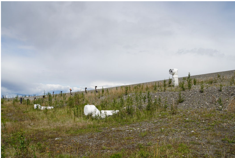
Figure 5-9 Air Convection Culverts at Beaver Creek, Yukon Territory, Canada (photo by B. Connor)
