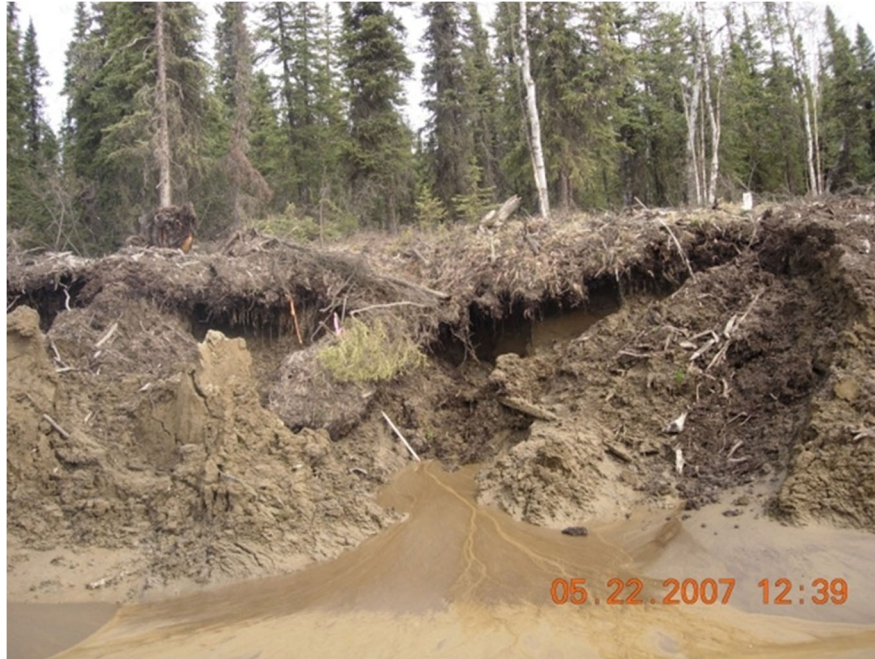
Figure 6-3 Advanced thaw degradation of cut slope shows block failures and runoff of highly fluid silt into ditch
