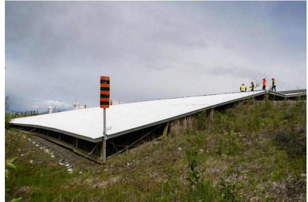
Figure 5-12 Snow Shed Installed near Beaver Creek Canada (Photo B. Connor)
