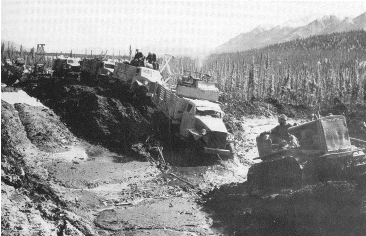
Figure 1-1 Thawing permafrost during the construction of the Alaska-Canadian Highway (Coates 1992).
