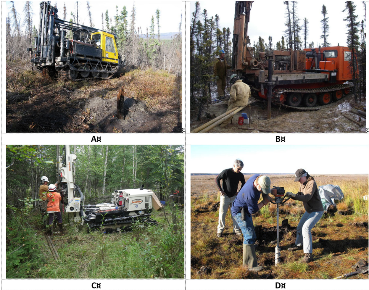
Figure 3-9 Drilling methods used for geotechnical studies in permafrost areas of Alaska. A – Drill rig performing solid-stem and hollow-stem drilling at the Dalton Highway Innovation Project field site, May 2008; operated by DOT&PF crew; equipped with a modified CME sampler (2 in. inside diameter); depth of drilling – up to 30 m; B – Drilling with a Nodwell mounted CME 55 drill rig with a 154 kg automatic hammer for split-spoon sampling at the HAARP field site, October 2007; performed by Discovery Drilling Inc. crew; depth of drilling – up to 20 m; C – Direct-push Geoprobe drilling performed by CRREL crew, CCHRC field site, August 2014; depth of drilling – up to 20 m; D – Drilling with the SIPRE corer, UAF AUTC project, field site AR-6, Anaktuvuk area, September 2010; SIPRE corer (7.5 cm inner diameter) was equipped with a small (1.89 cu. in., 1.3 h.p.) two-stroke Tanaka TIA-340 engine; depth of drilling – up to 6 m.
