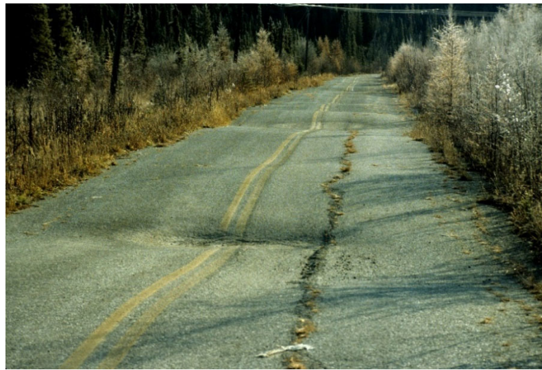
Figure 7-8 Thawing of deep ice wedges on the abandoned section of the Richardson Highway east of Fairbanks
