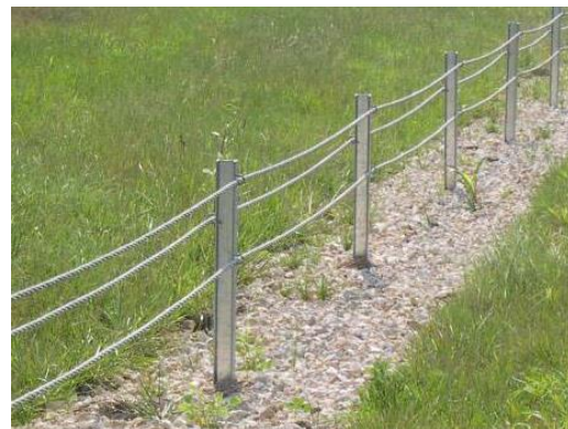
Figure 1.1: In-service three-strand, low-tension cable barriers in North Carolina
