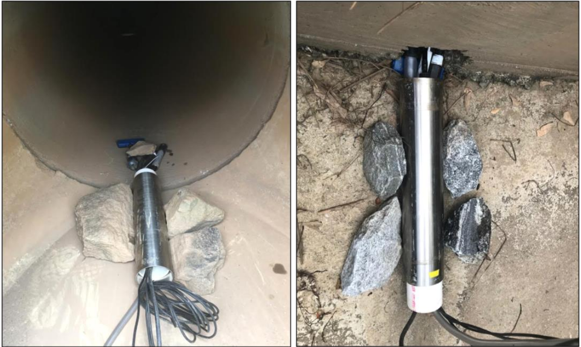
Figure 7. Photos. Test set-up for stormwater monitoring at BMP inflow and outflow.
