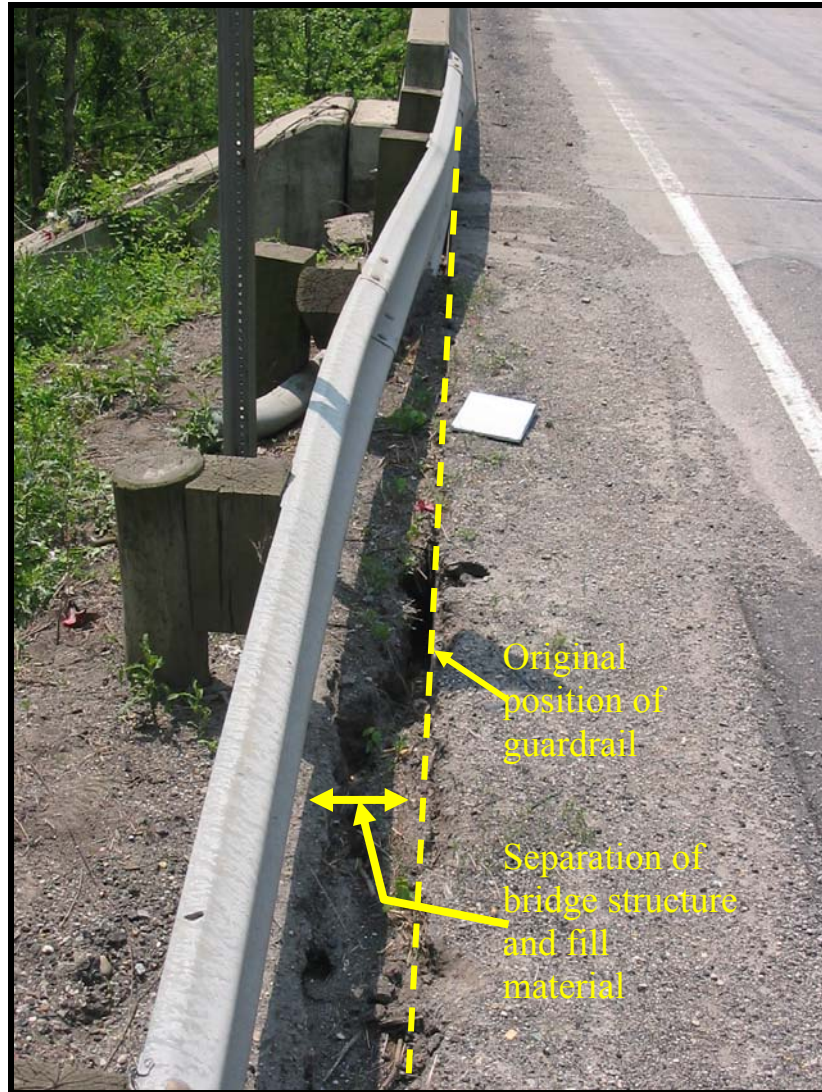
Figure 4.3 Separation between embankment and bridge structure
