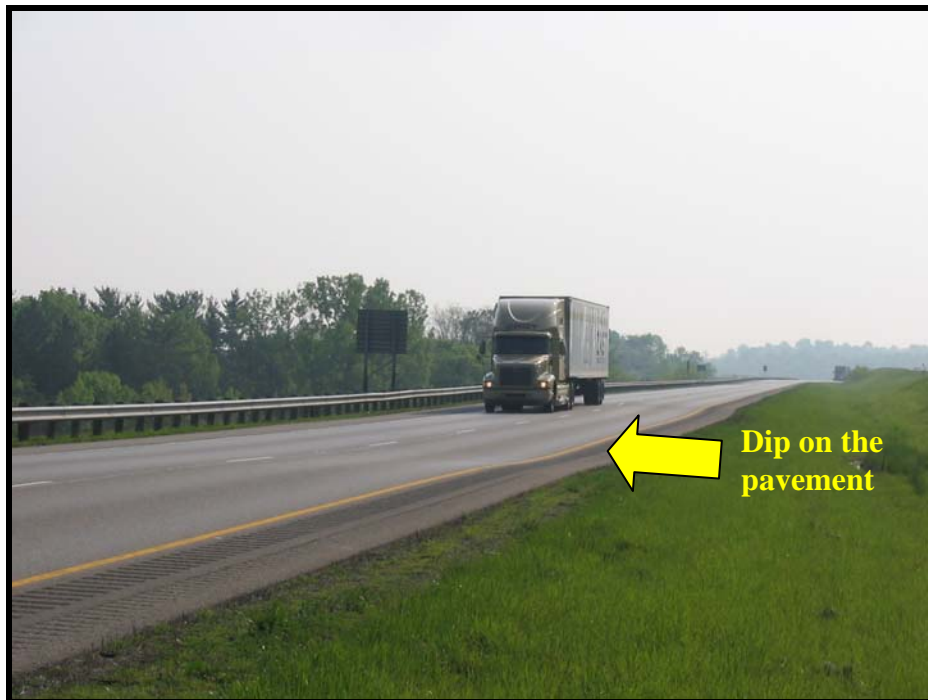
Figure 3.10 Roadway undulation/dip, receiving a risk score of 81
