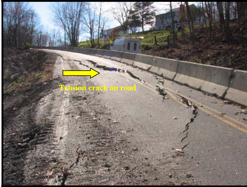
Figure 2.5 Tension cracks on road
