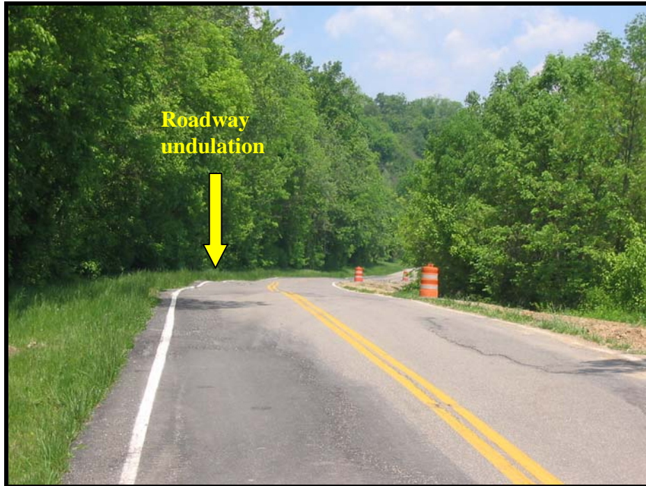
Figure 3.9 Roadway undulation/dip, receiving a risk score of 81
