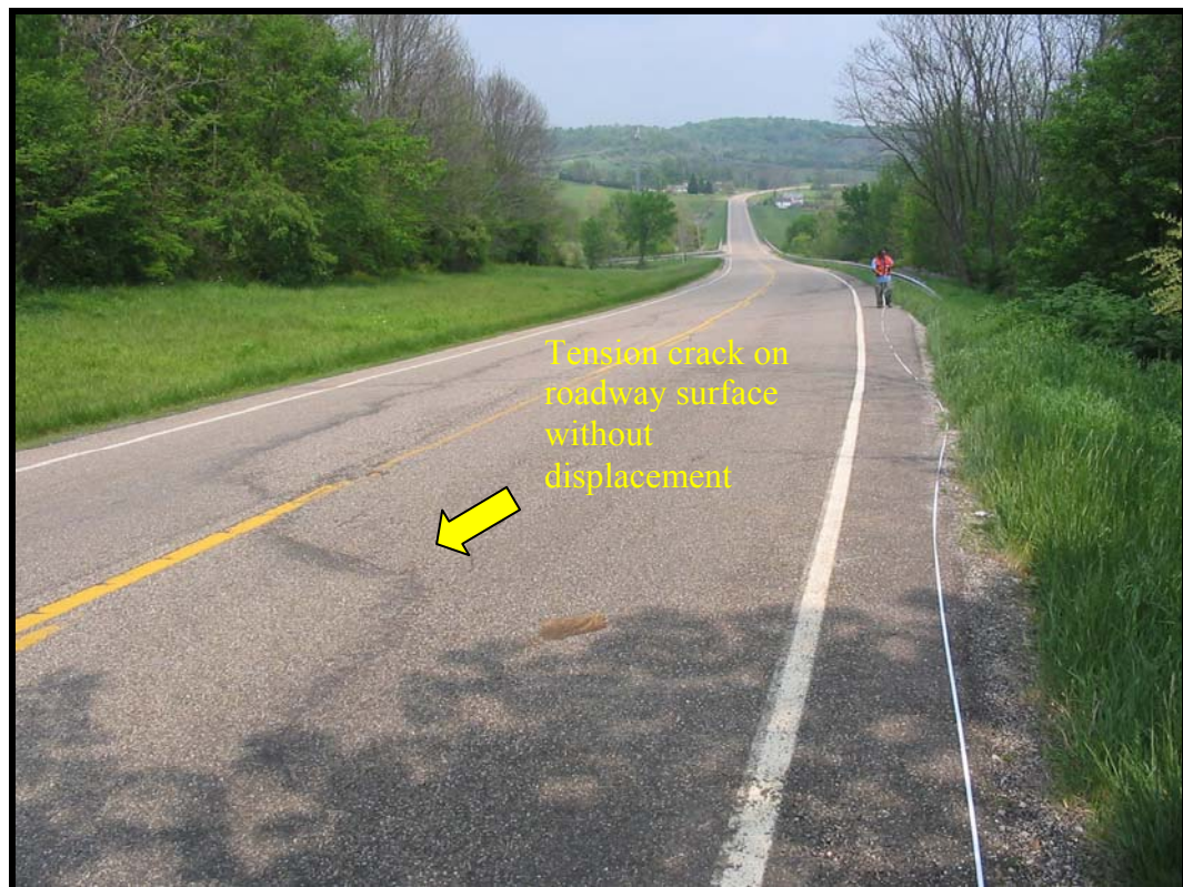
Figure 4.11 Crack line on pavement
