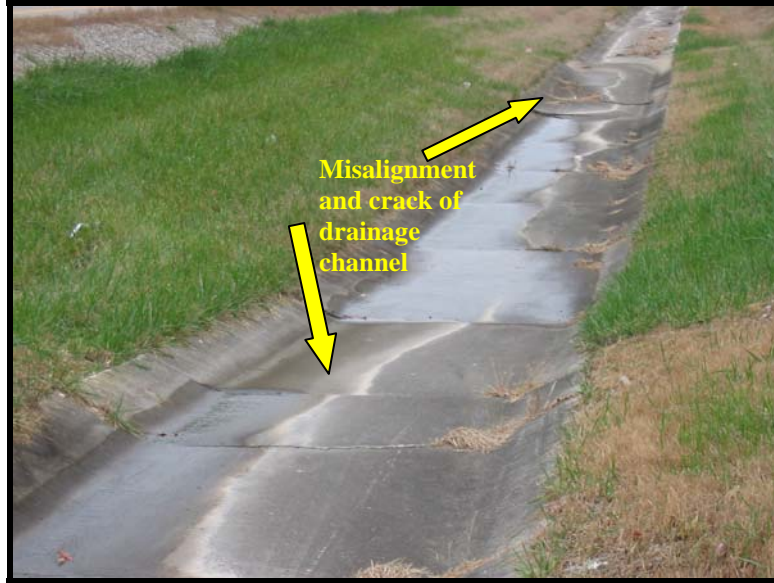
Figure 2.3 Misalignment of drainage channel
