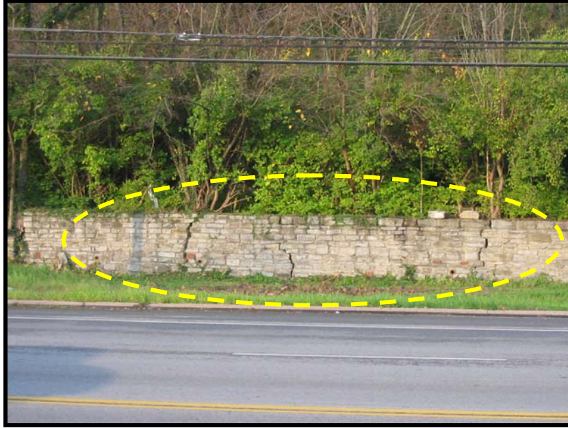
Figure 2.7 Failure of earth retaining structure
