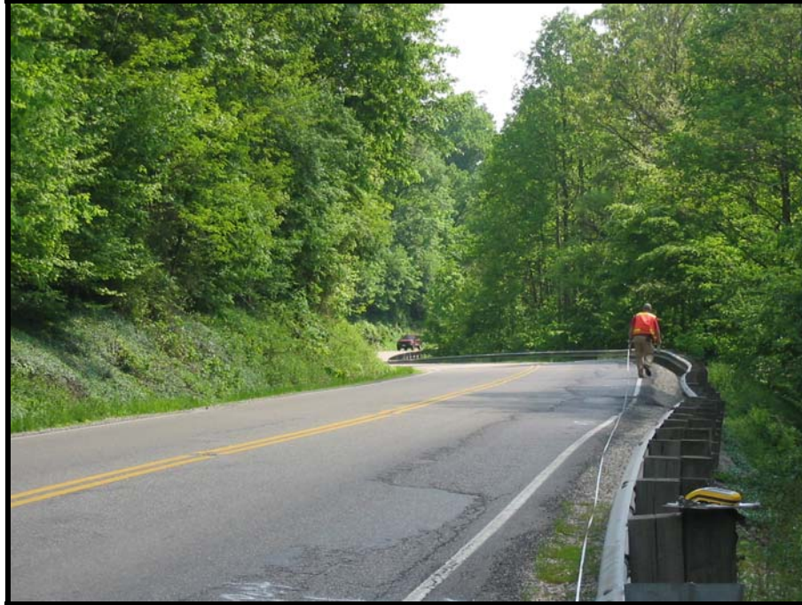
Figure 3.17 Example of a horizontal curve that could hide the slope hazard on the road ahead
