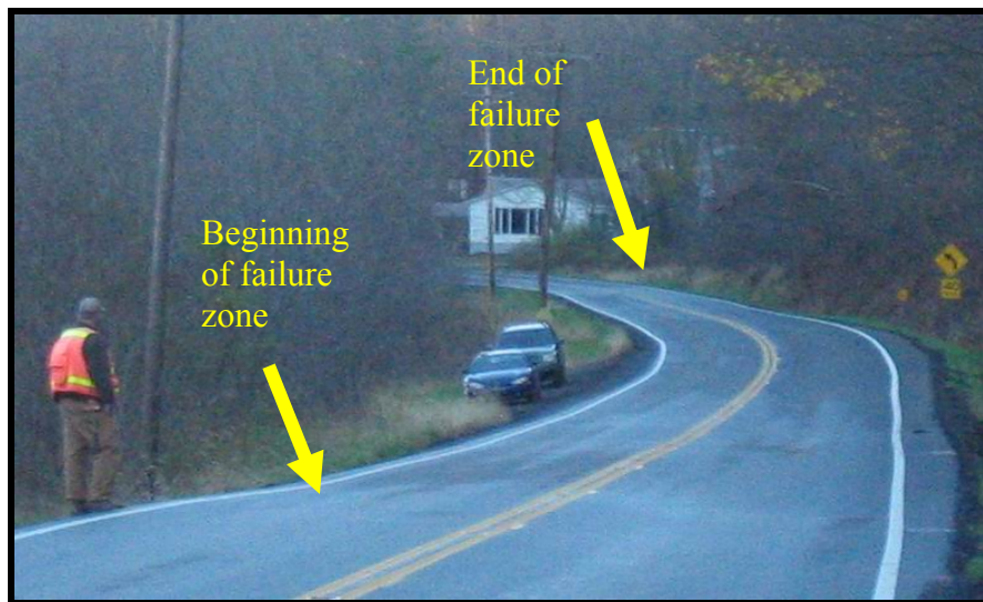
Figure 3.13 Newly paved roadway surface with evidence of failure that may not be obvious to the investigator
