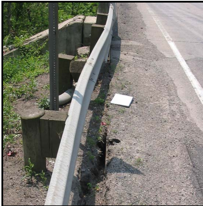
Figure 3.11 Separation of the slope and a bridge structure
