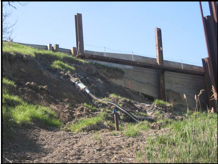
Figure 3.12 Effect of a slope failure to the stability of a bridge structure that requires immediate response
