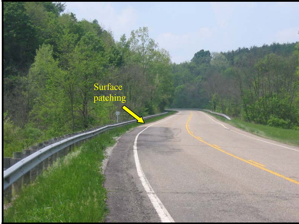
Figure 4.12 Surface patching and transverse cracks
