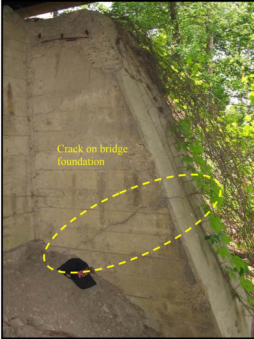
Figure 4.4 Cracks at the bridge foundation
