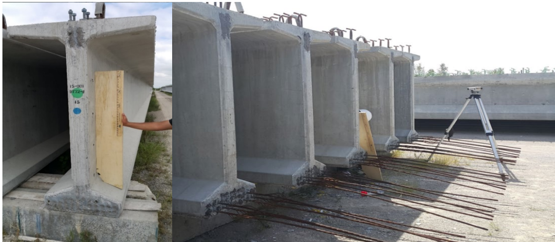
Figure 3-8. Automatic level with wooden template used to measure camber of the bottom flanges.
