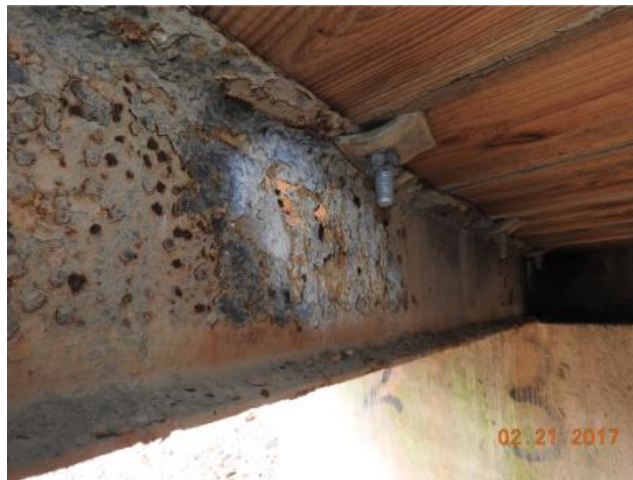
Figure 15. Example of Steel Beam Timber Deck Web Corrosion
