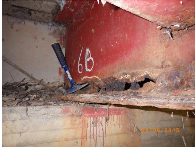
Figure 1. Example of Extensive Beam End Corrosion Damage
