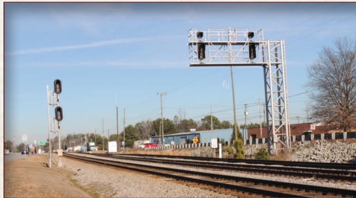
Automatic block signals, Fairburn vicinity (Fulton County)
