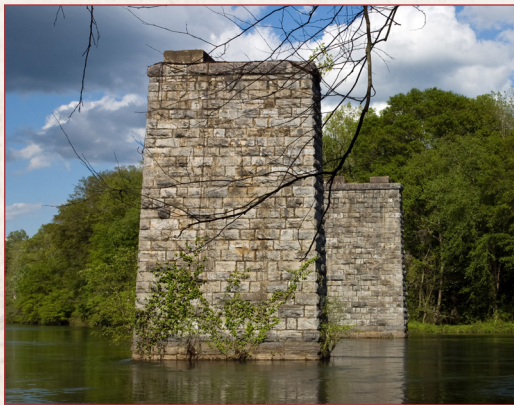
Ashlar stone piers of Western & Atlantic's old Etowah River bridge (Bartow County)
