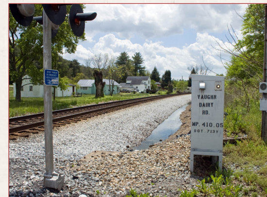
Signal box for crossing signal at Vaughn Dairy Road in Rydal (Bartow County)
