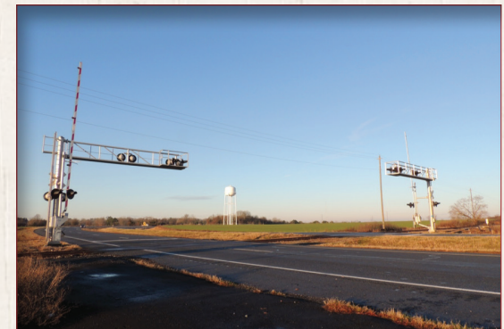
Typical grade crossing signal with gate and mast arm, Fort Valley (Peach County)
