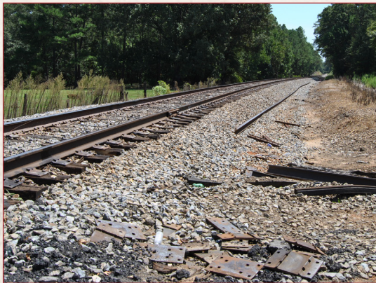
Disposed tie plates alongside tracks at Bucks in Fort Valley vicinity (Peach County)
