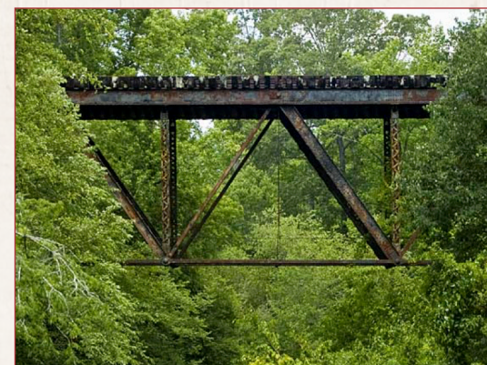
Warren type deck-truss bridge at Hard Labor Creek near Apalachee (Morgan County)
