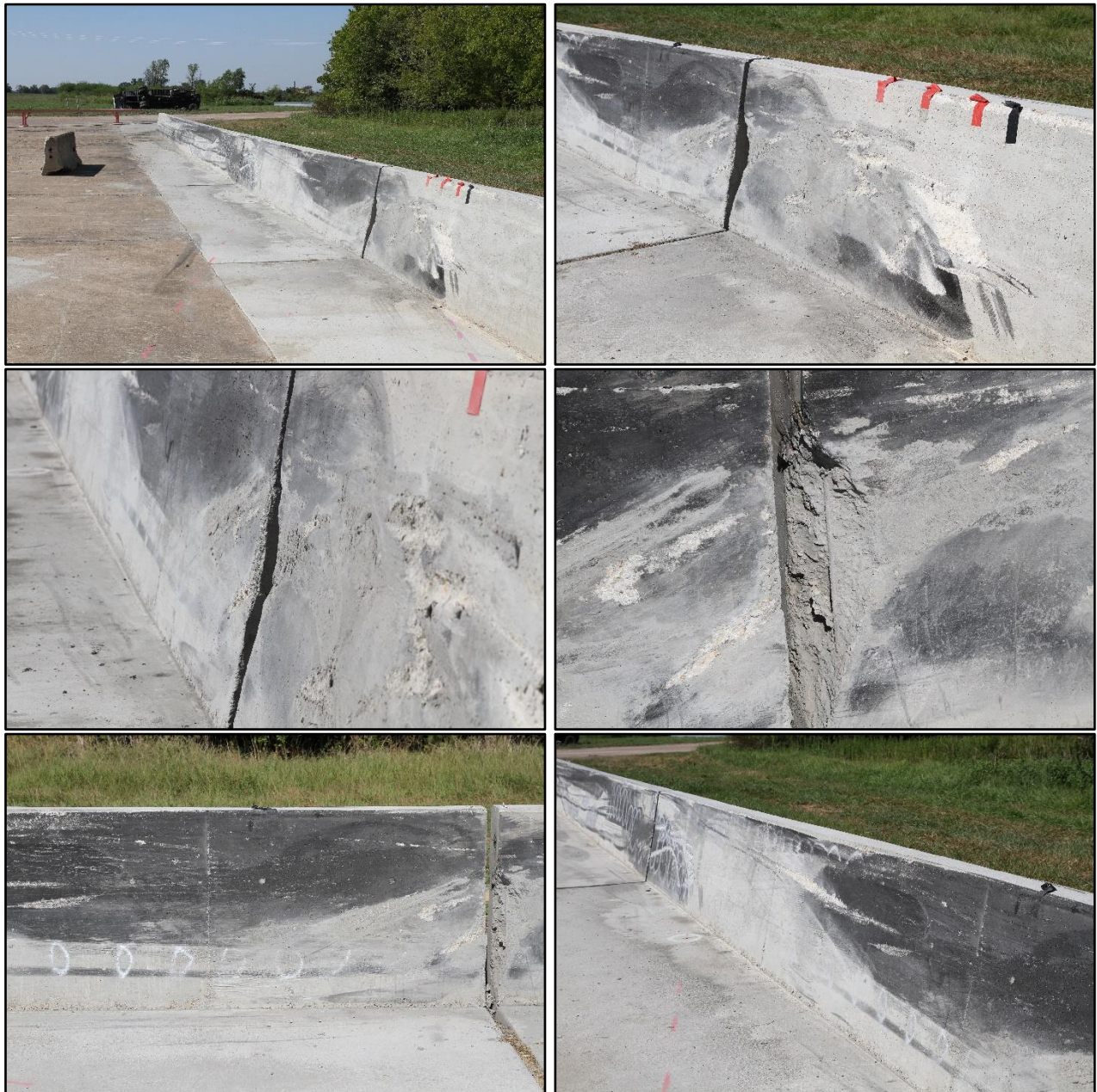
Figure 7.4. TxDOT Shallow Anchorage SSSTR without Dowel Bars and with Concrete Apron Extended Downstream of Barrier after Test No. 469680-02-3.
