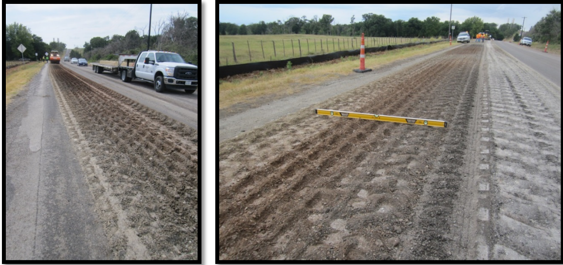
Figure 48. Material Variability on SH 7.
