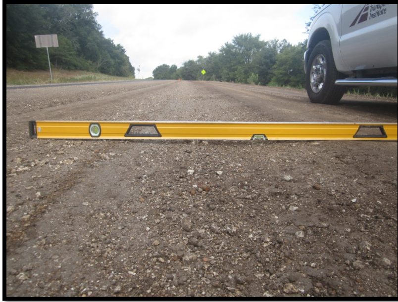
Figure 46. Instability in Location Constructed at Excessive Moisture.
